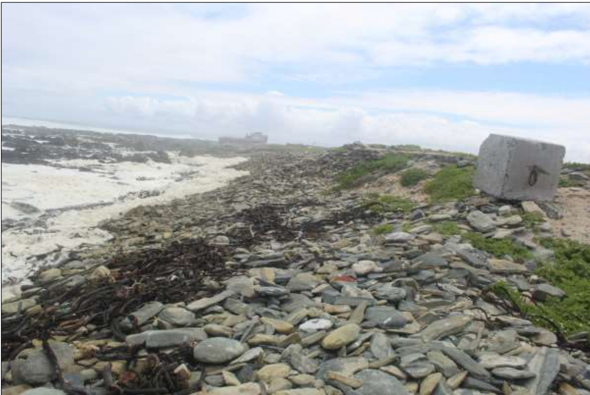
Northern section of the main wall, side facing the sea, close view north.
