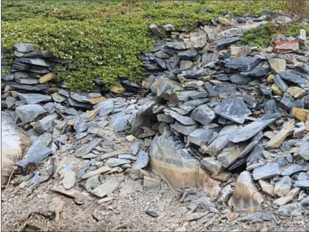
Wall 10, generally collapsed.
