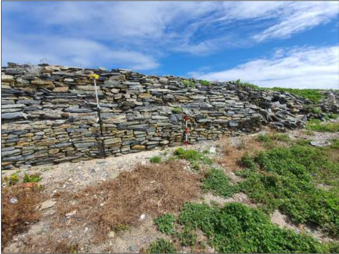
Wall 3a, west of collapse.
