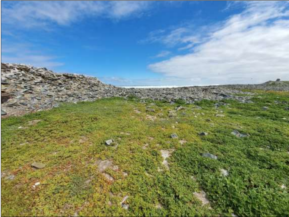
Collapsed mid-section of the main wall.
