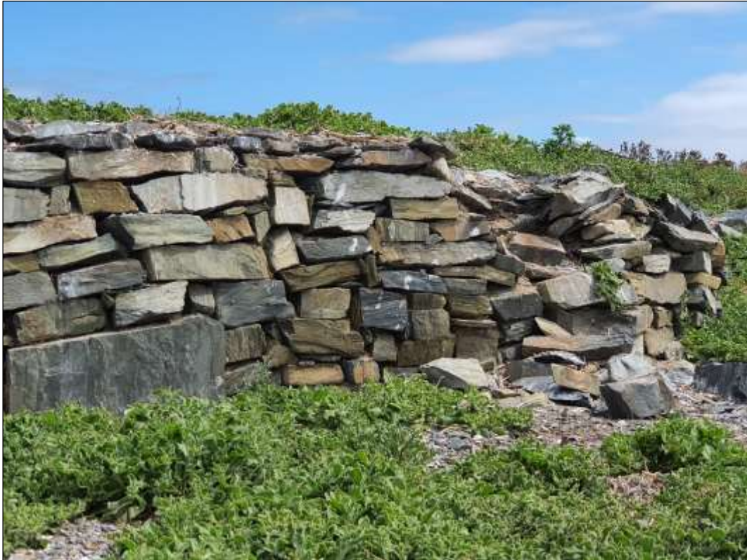
Wall 2a, shows bulge and toppling.
