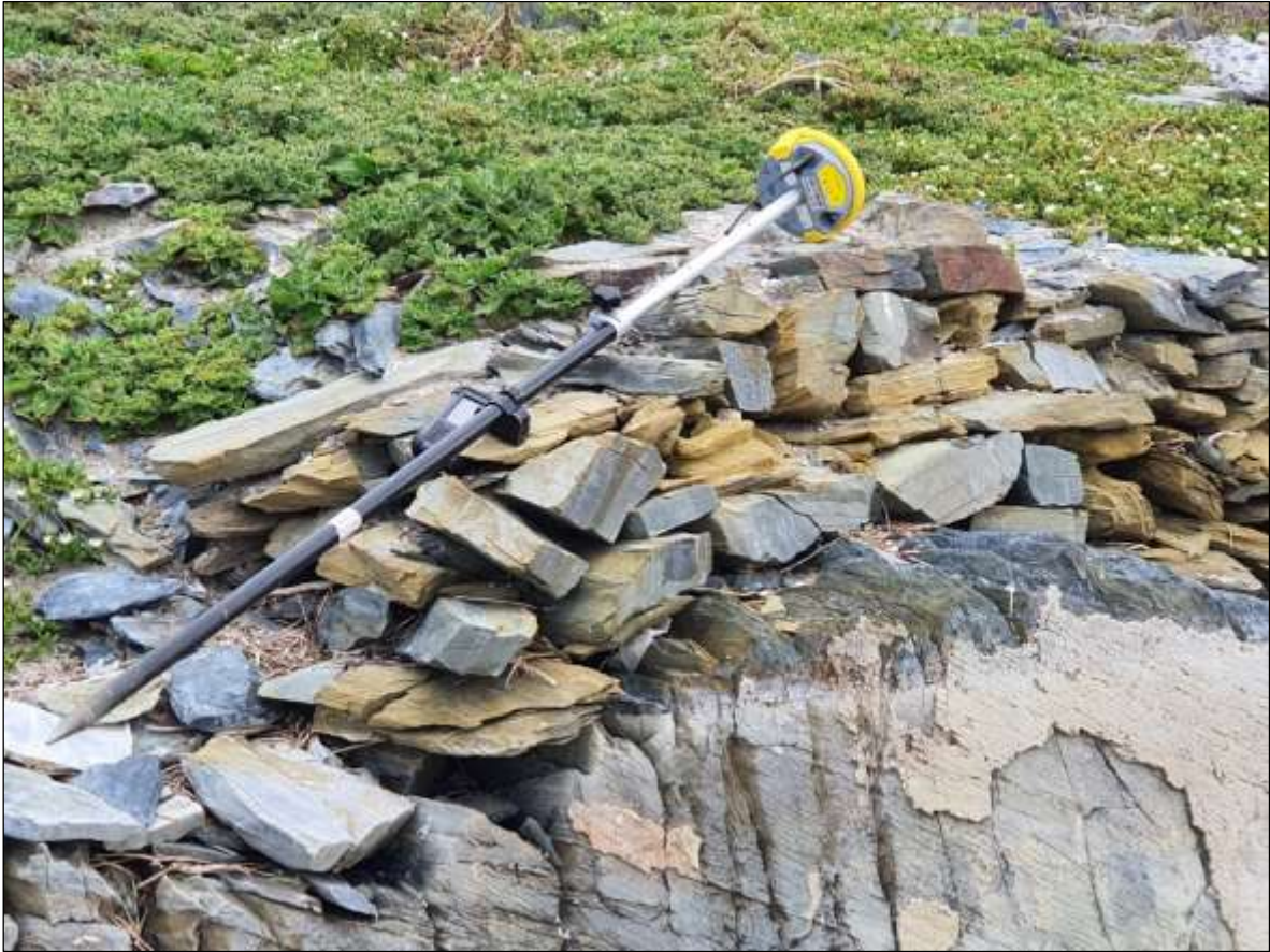
Wall 12, terrace wall, with collapsed ends.
