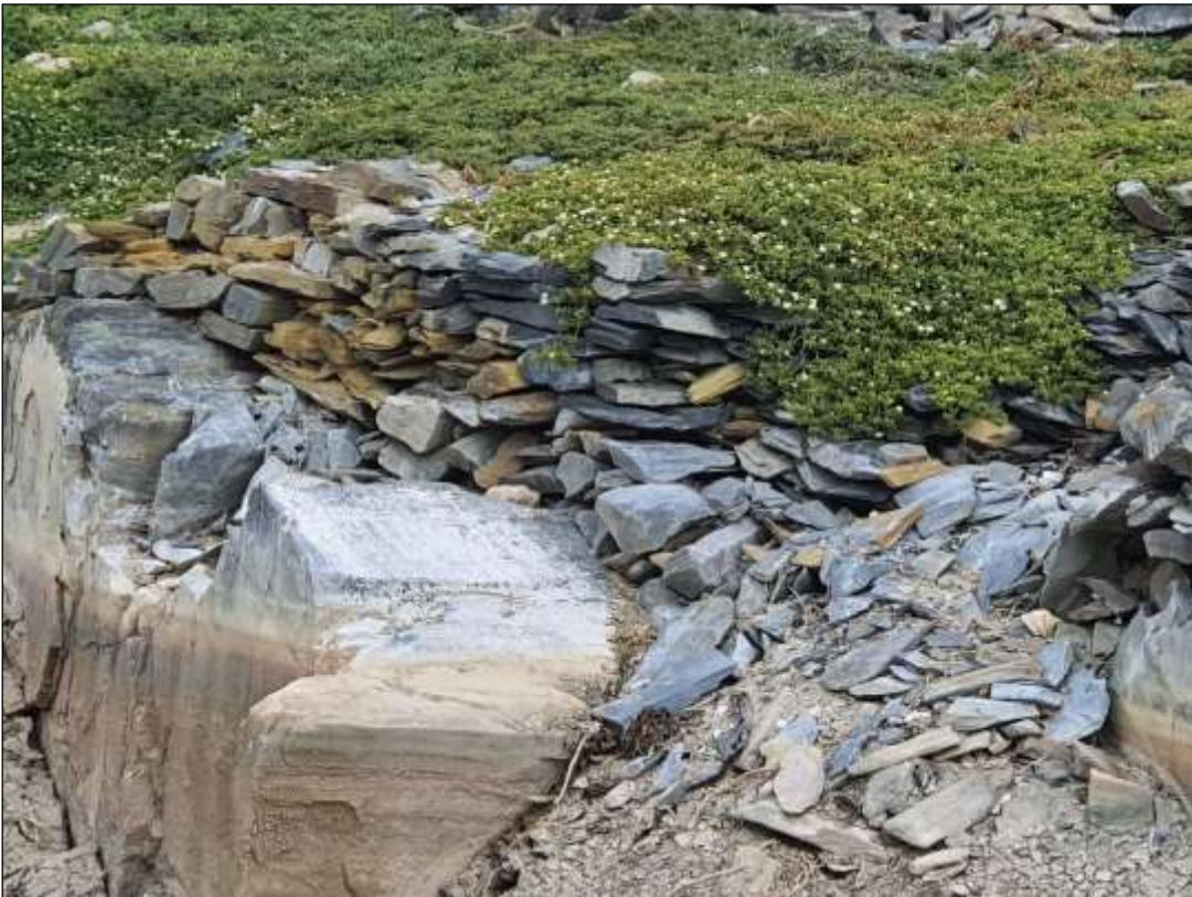
Wall 11, partially collapsed.
