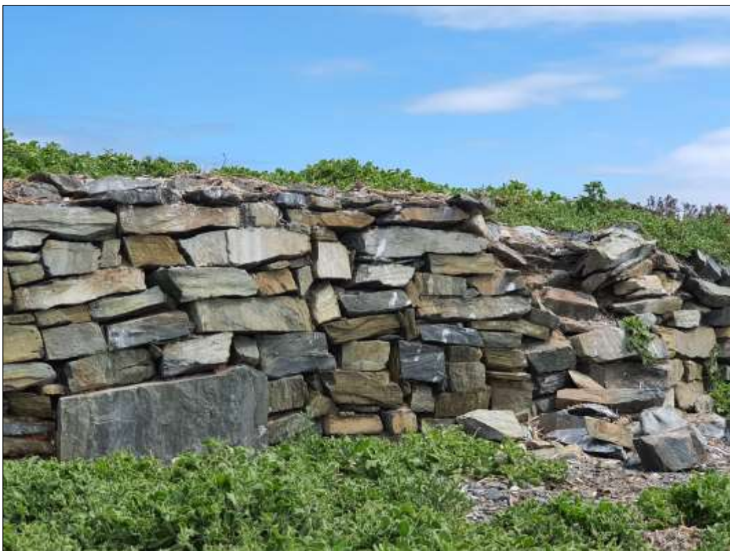
Wall 2b west (right side) of bulge.
