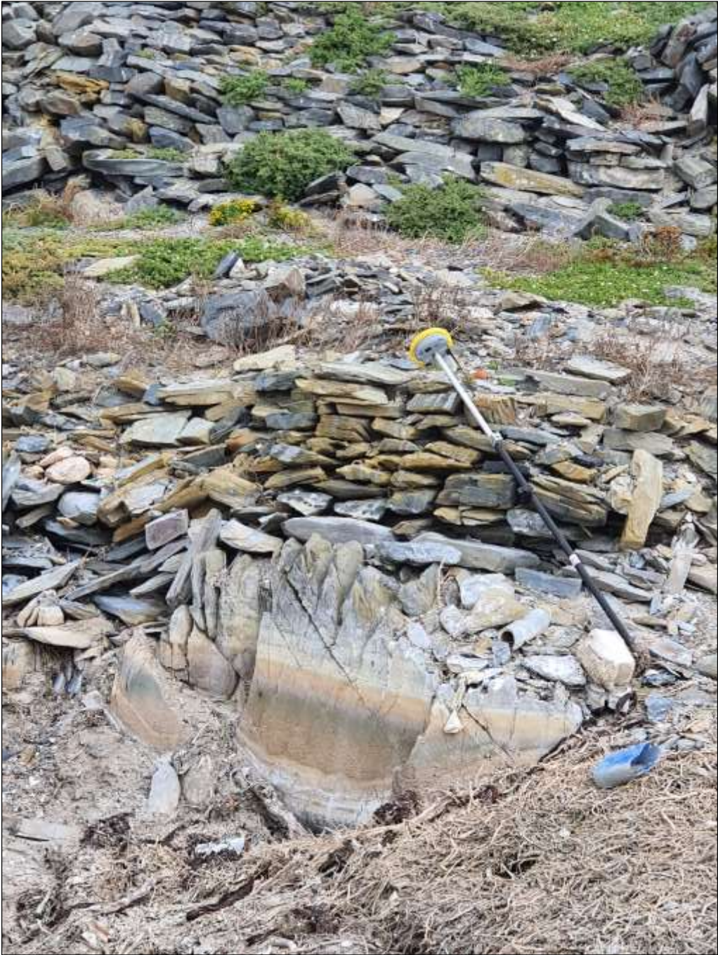
Wall 9 with collapsed ends.
