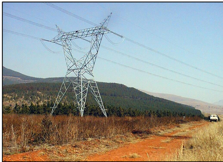
Figure 3: Self-Supporting Strain Tower
