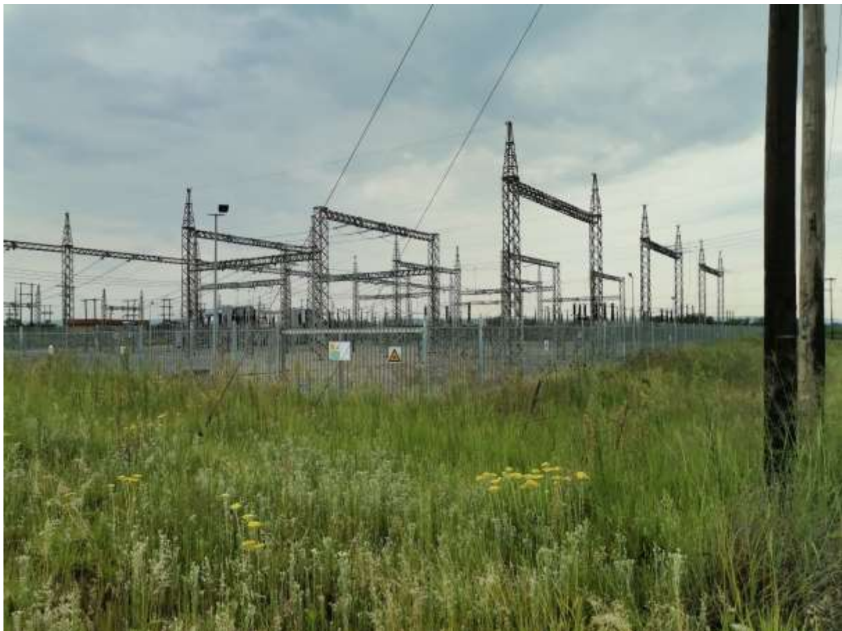
Figure 27: Eskom Roan Substation in very close proximity to the proposed project.
