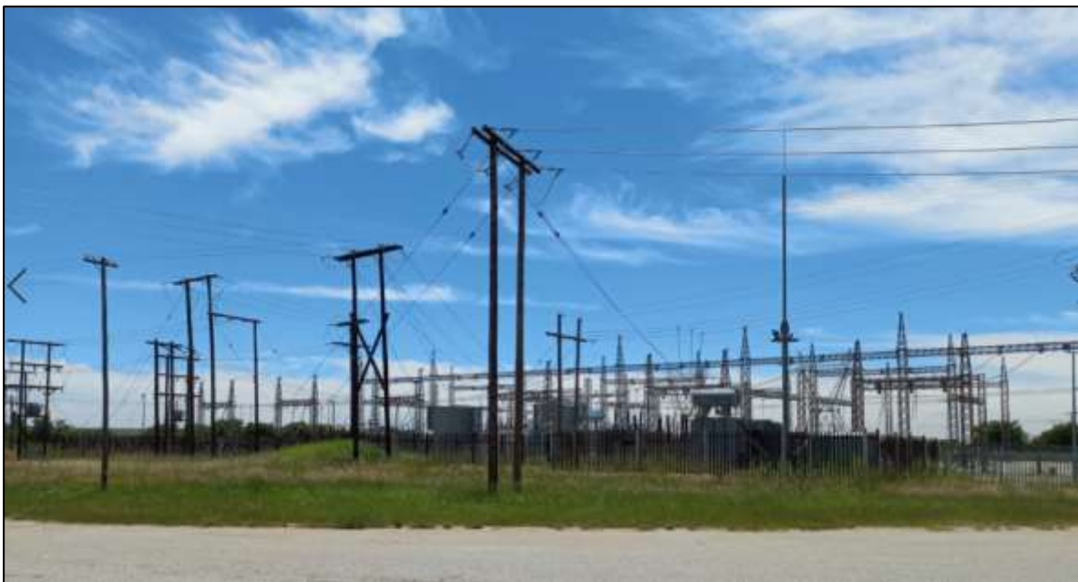
Figure 59: Photograph of Rietkuil Substation (Stead, 2022)
