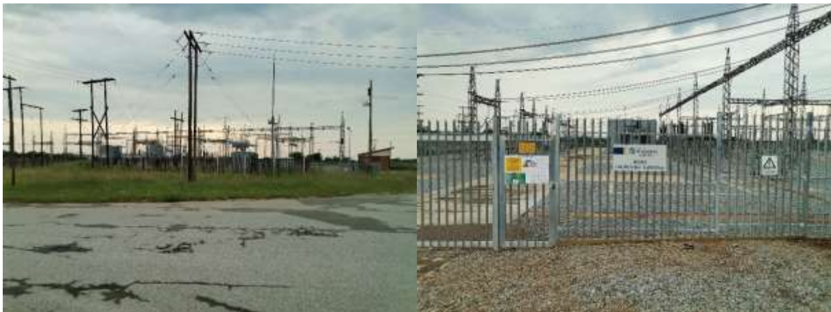
Figure 13: Existing Eskom Roan Substation to which the project will connect.
