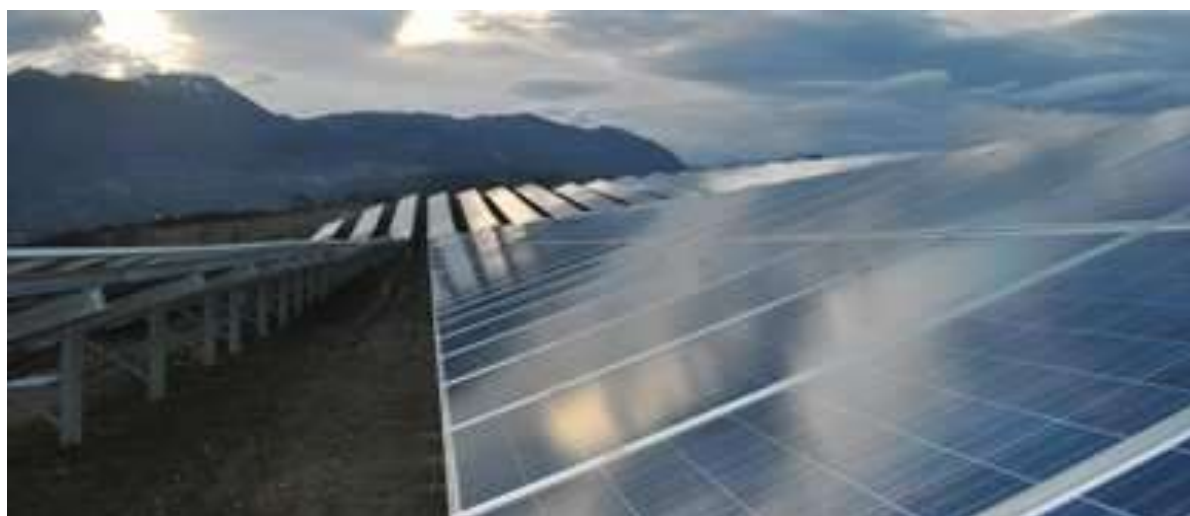
Figure 9: Photographic example of rack or fixed structure (AMDA Developments, 2022)
