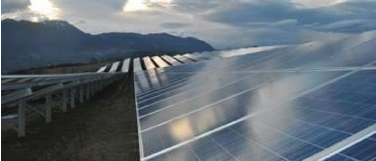
Figure 8: Photographic example of rack or fixed structure (AMDA Developments, 2022)
