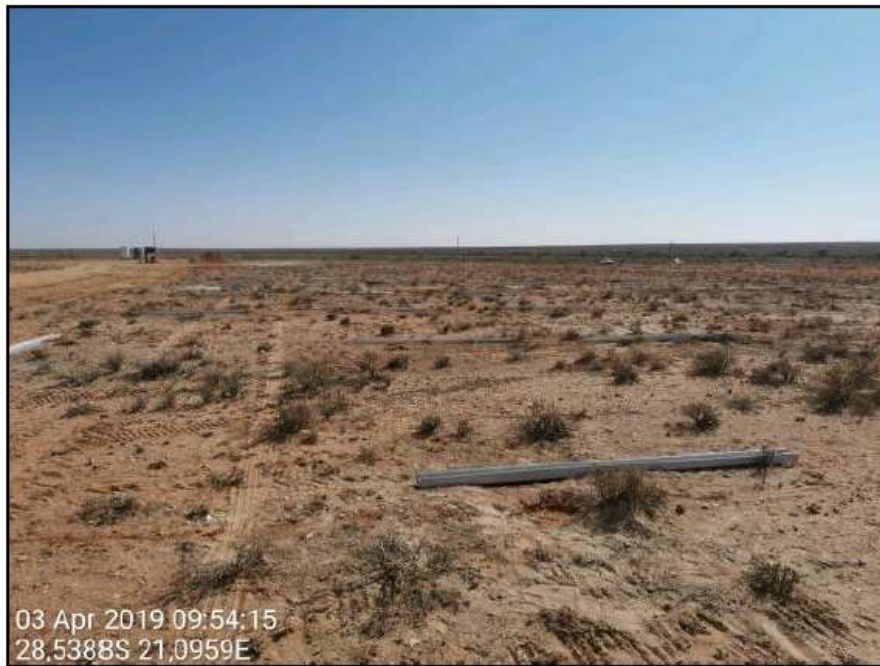
Figure 4: pre-drilled holes are backfilled with a wet sand mixture and steel piles placed in position ready for ramming.
