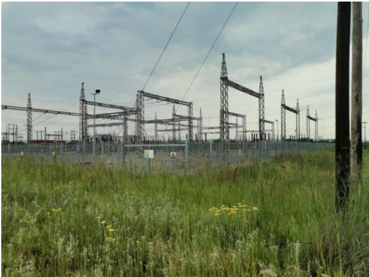
Figure 25: Eskom Roan Substation in very close proximity to the proposed project.
