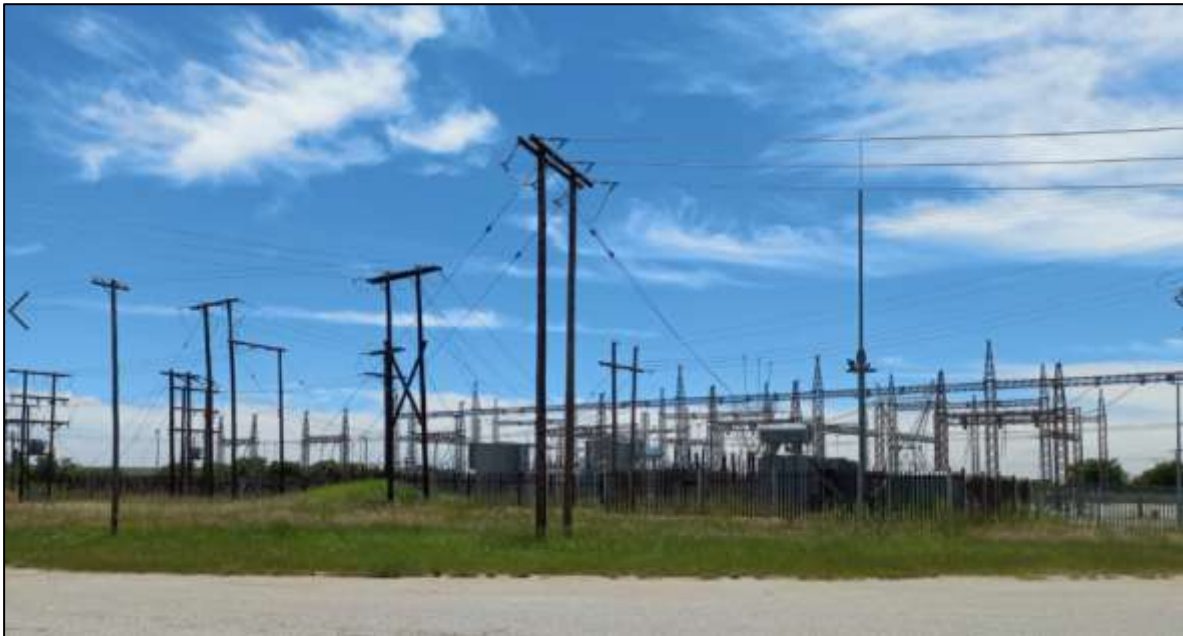
Figure 58: Photograph of Rietkuil Substation (Stead, 2022)
