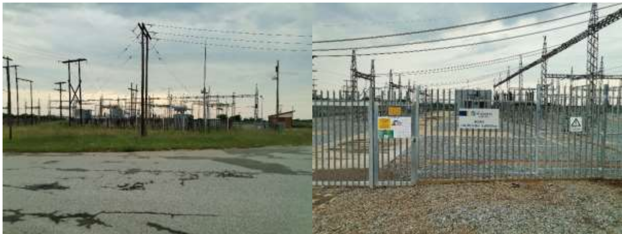
Figure 12: Existing Eskom Roan Substation to which the project will connect.
