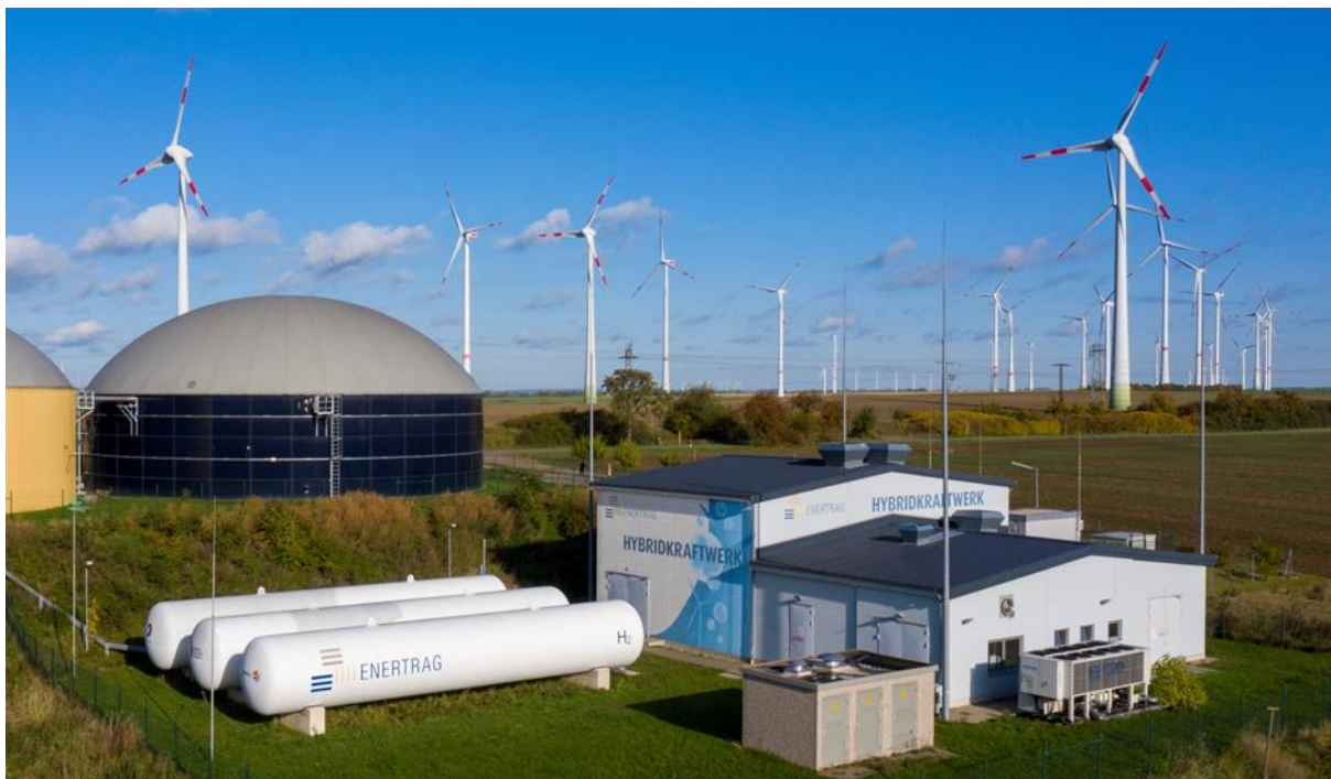
Figure 6-4: Closer View of Electrolyser Housing and Storage Tanks
