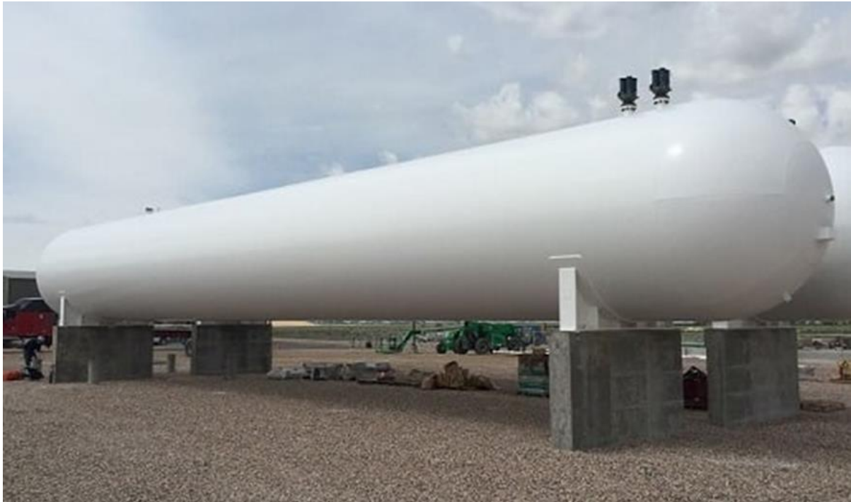
Figure 6-17: Bullet storage tank (ammonia/hydrogen storage)
