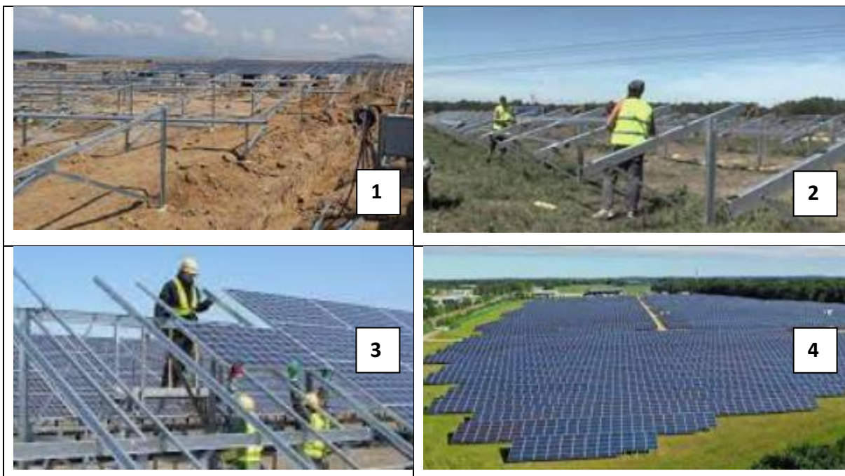
Figure 17: Illustration of the construction process in solar farms (construction progress indicated from 1 to 4)
