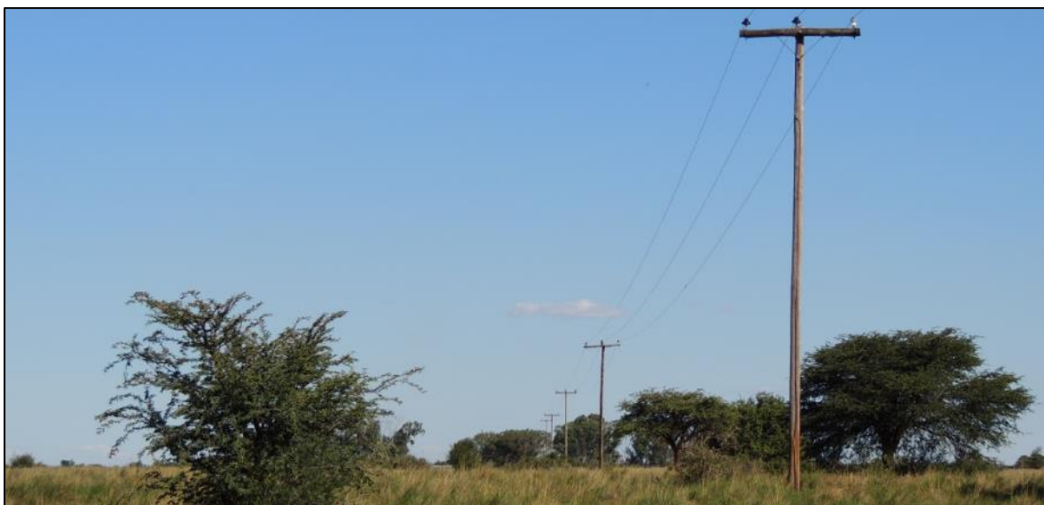
Figure 45. Acacia type thorn trees adding to the local sense of place (Stead, 2022)
