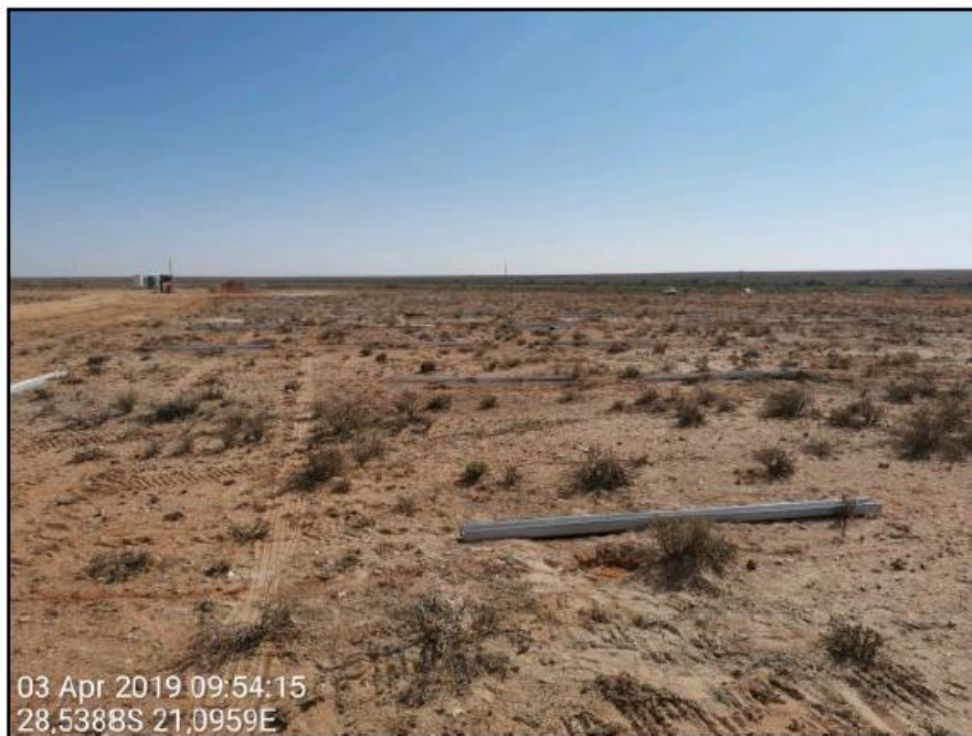
Figure 5: pre-drilled holes are backfilled with a wet sand mixture and steel piles placed in position ready for ramming.
