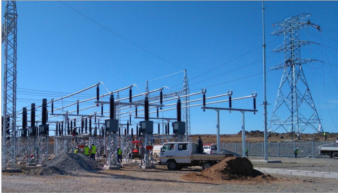
Figure 22: Example of High Voltage Transmission Line Connecting to Substation
