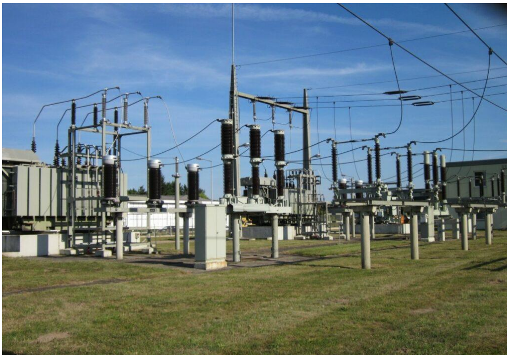
Figure 14: Example of High Voltage Substation (source: https://www.protoenergy.com/ )
