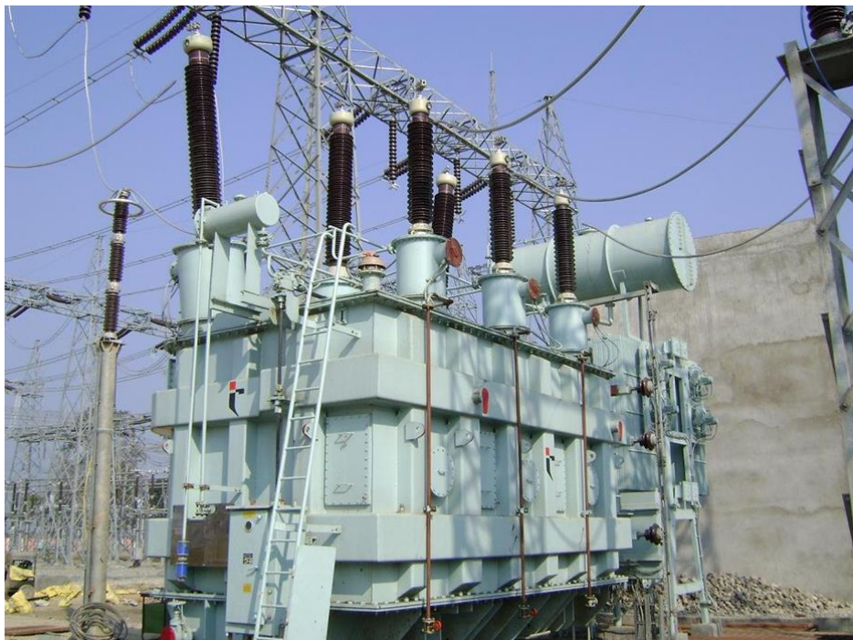
Figure 13: Example of Medium Voltage Transformer (source: https://www.ulaginoli.com/ )
