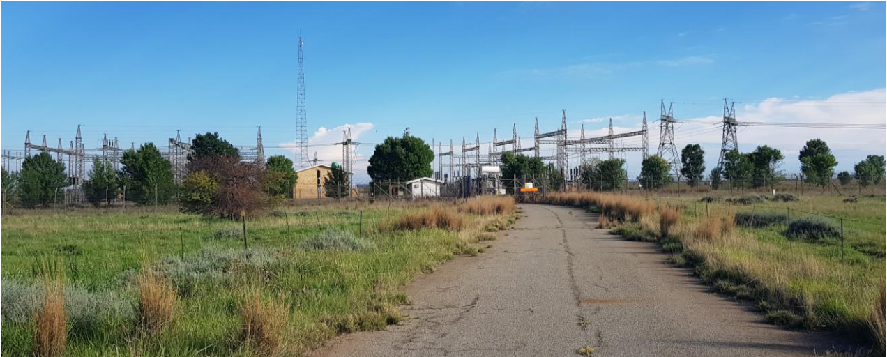
Figure 18: Northern view of the Jersey Distribution Substation
