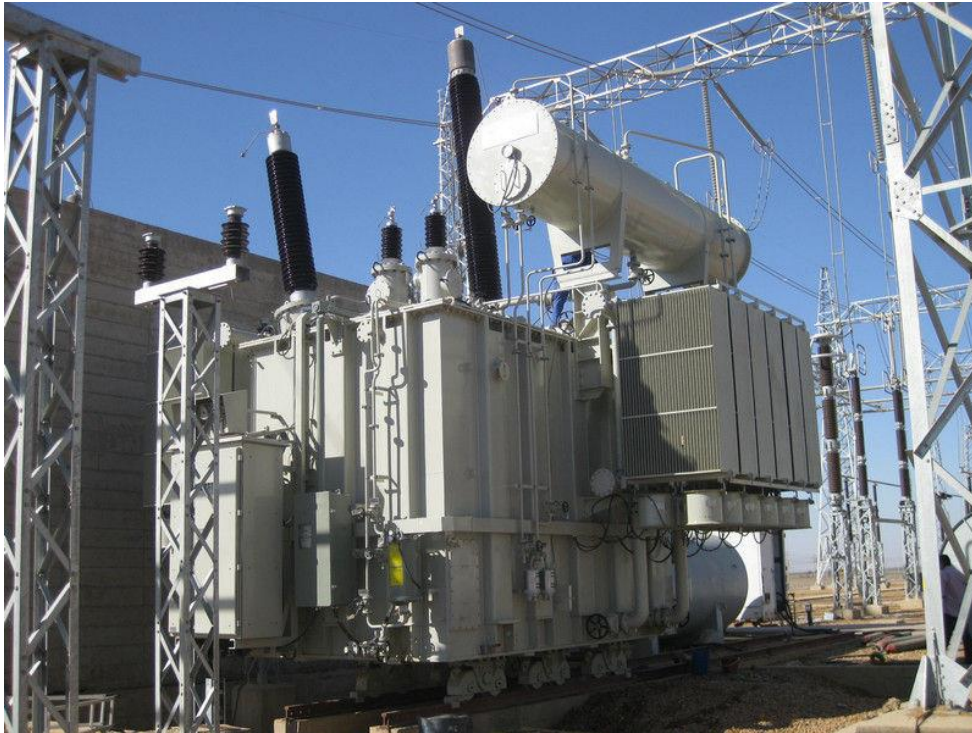
Figure 15: Example of High Voltage Transformers
