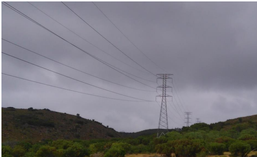
Figure 17: Example of a 132 kV transmission line
