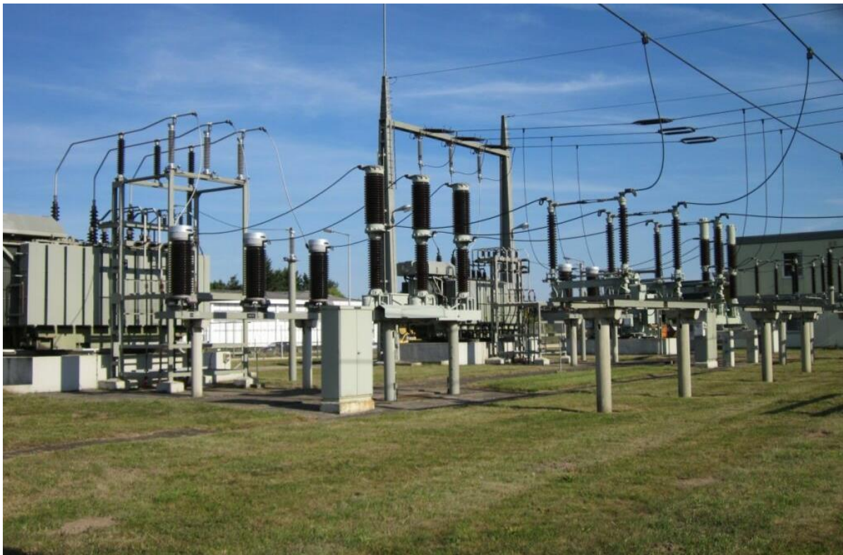
Figure 12: Example of High Voltage Substation (source: https://www.protoenergy.com/ )
