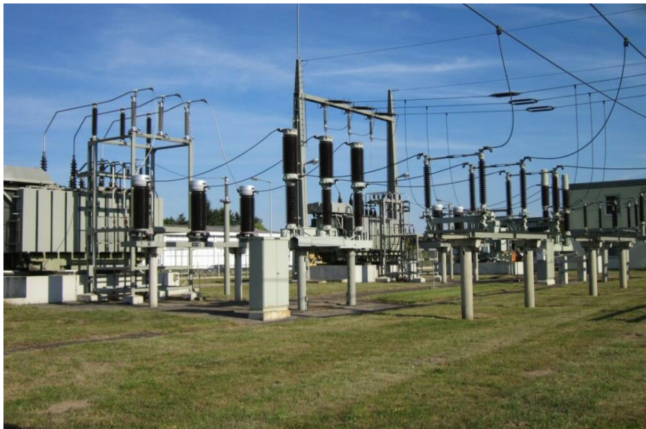
Figure 12: Example of High Voltage Substation
