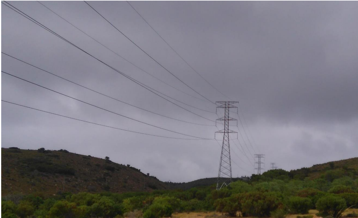
Figure 17: Example of a 132 kV transmission line
