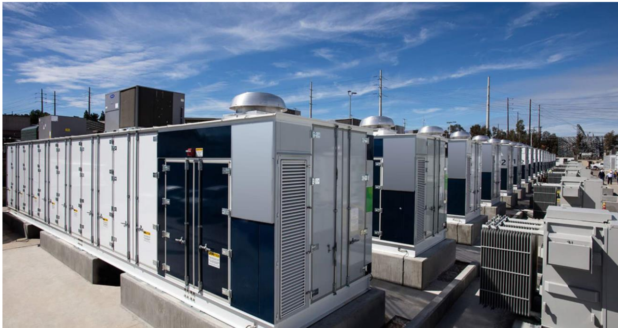
Figure 16: Example of BESS installation ( https://biiworld.com/ )
