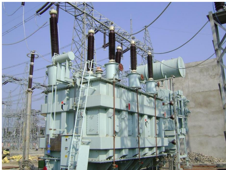
Figure 11: Example of Medium Voltage Transformer (source: https://www.ulaginoli.com/ )
