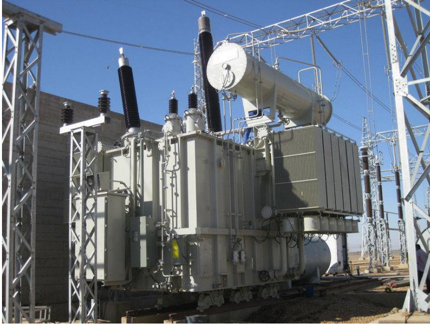
Figure 13: Example of High Voltage Transformers (source: https://www.electricityforum.com/ )
