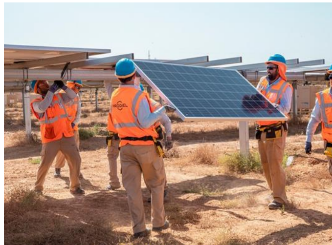
Figure 2-7: Photographs depicting the construction phase of a solar farm similar to De Rust PV1 SEF. Source: www.power-technology.com , renewablesnow.com .
