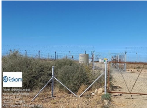
Figure 2-4: Entrance to Kronos substation
