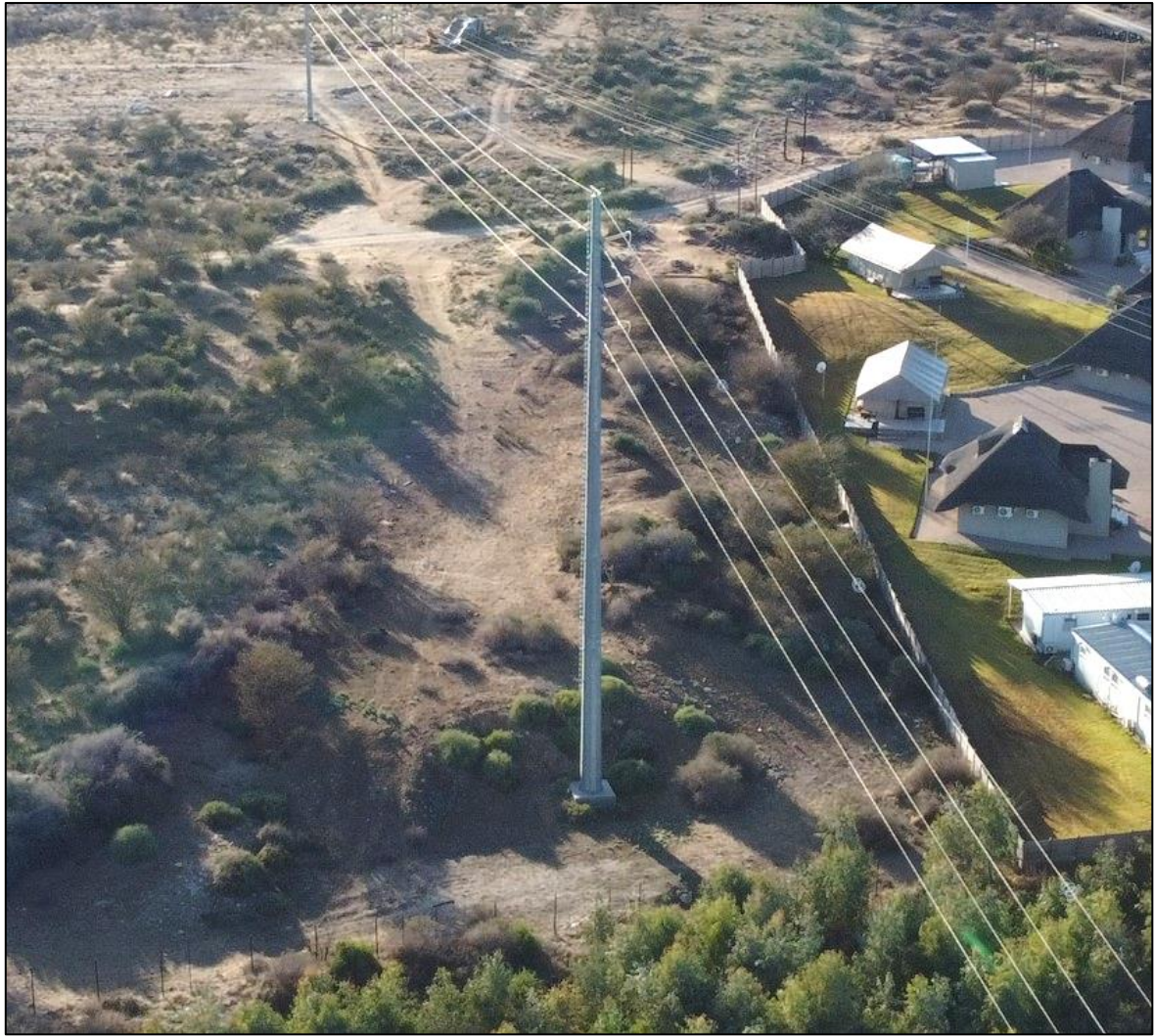
Figure 3: An aerial photograph of the existing 132 kV transmission line's pylon. Note the vegetation growing around this pylon, indicating the minimal disturbance required for the instalment of such structures. The small service road is also visible in this view.
