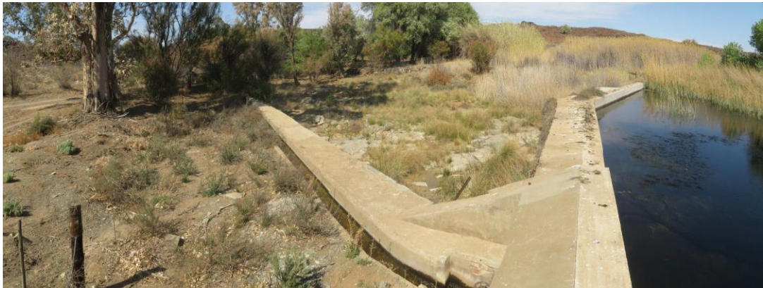
Figure 6-7: Functional weir in the Die Leegte River
