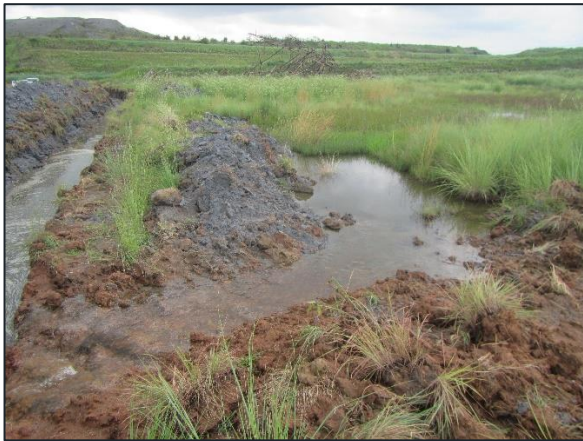
Figure 7-45 - Drainage channels that have been excavated by power station management to prevent the flooding of access roads
