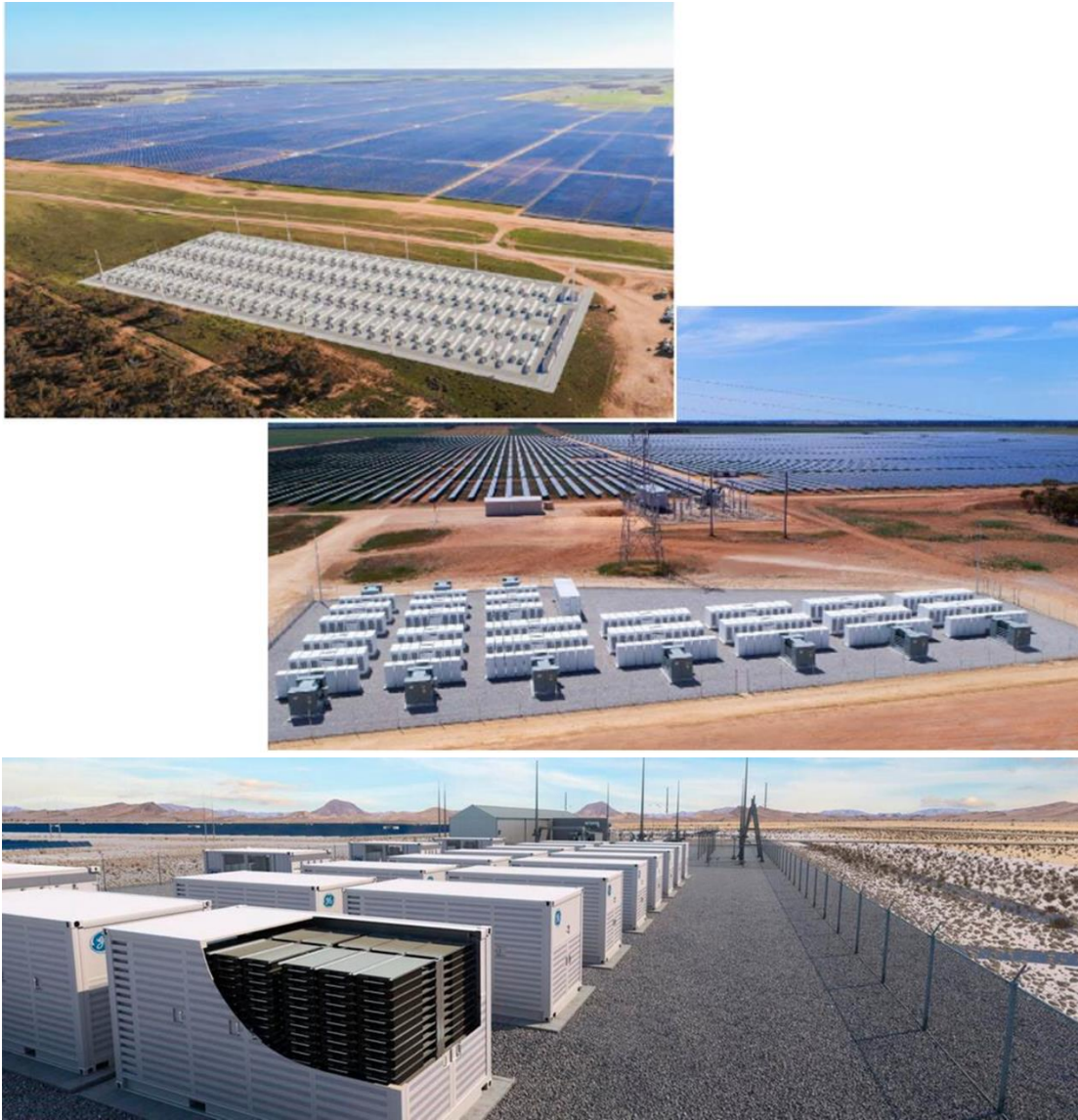
Figure 4-3 – Images of Typical BESS Systems
