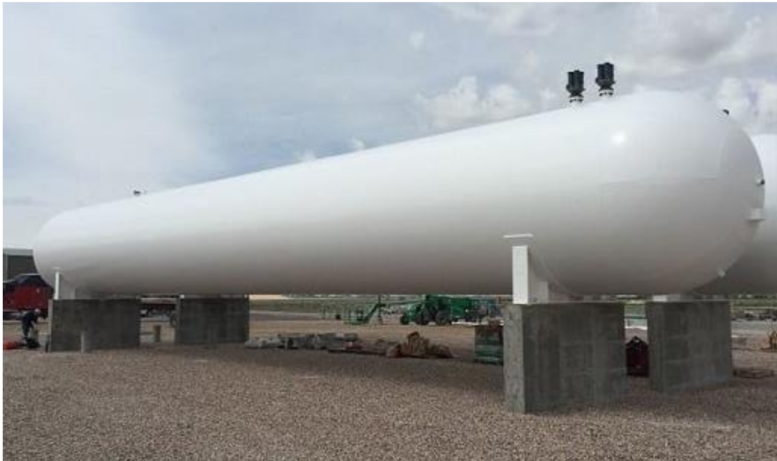
Figure 2-15: Bullet storage tank (ammonia storage)
