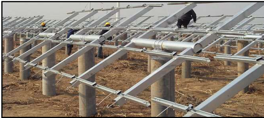
Figure 13 Support structure for Tracking PV Panels
