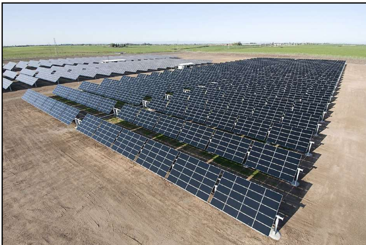
Figure 11 An Array of PV Panels once Mounted
