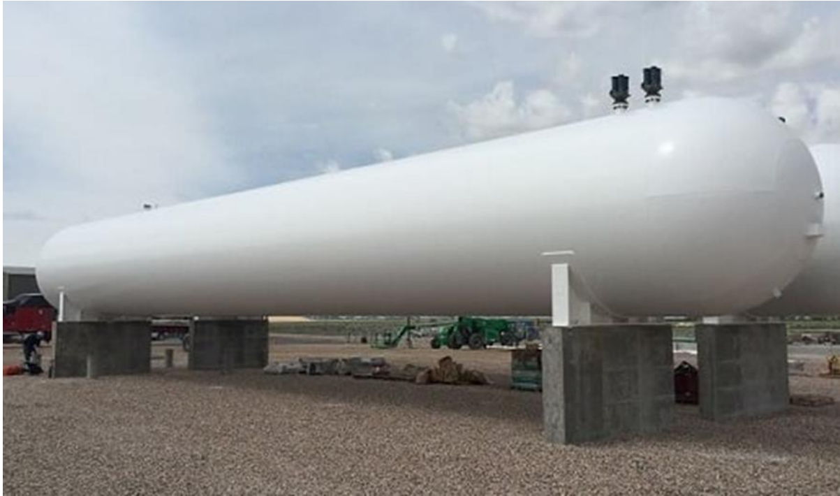
Figure 6-17: Bullet storage tank (ammonia/hydrogen storage)
