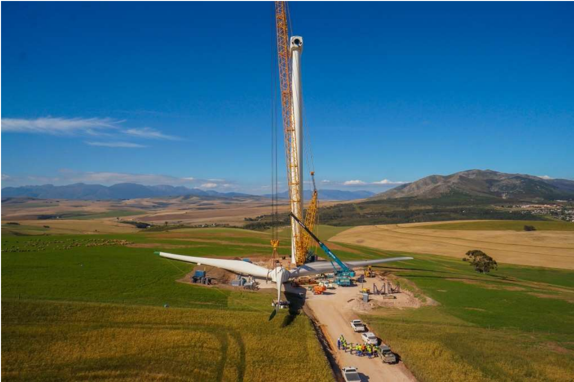
Figure 4-4: Construction of the Turbine – Preparing to lift the Rotor (Source: BioTherm Energy, 2016)
