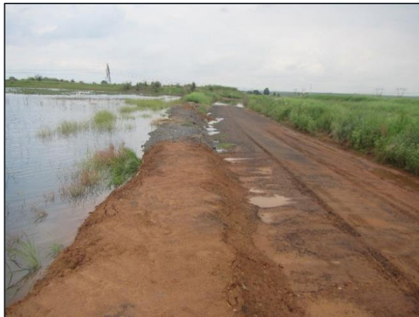
Figure 7-27: Amongst other features, gravel roads and drainage trenches have fragmented habitat in the local study area, and facilitated alien invasive species colonisation
