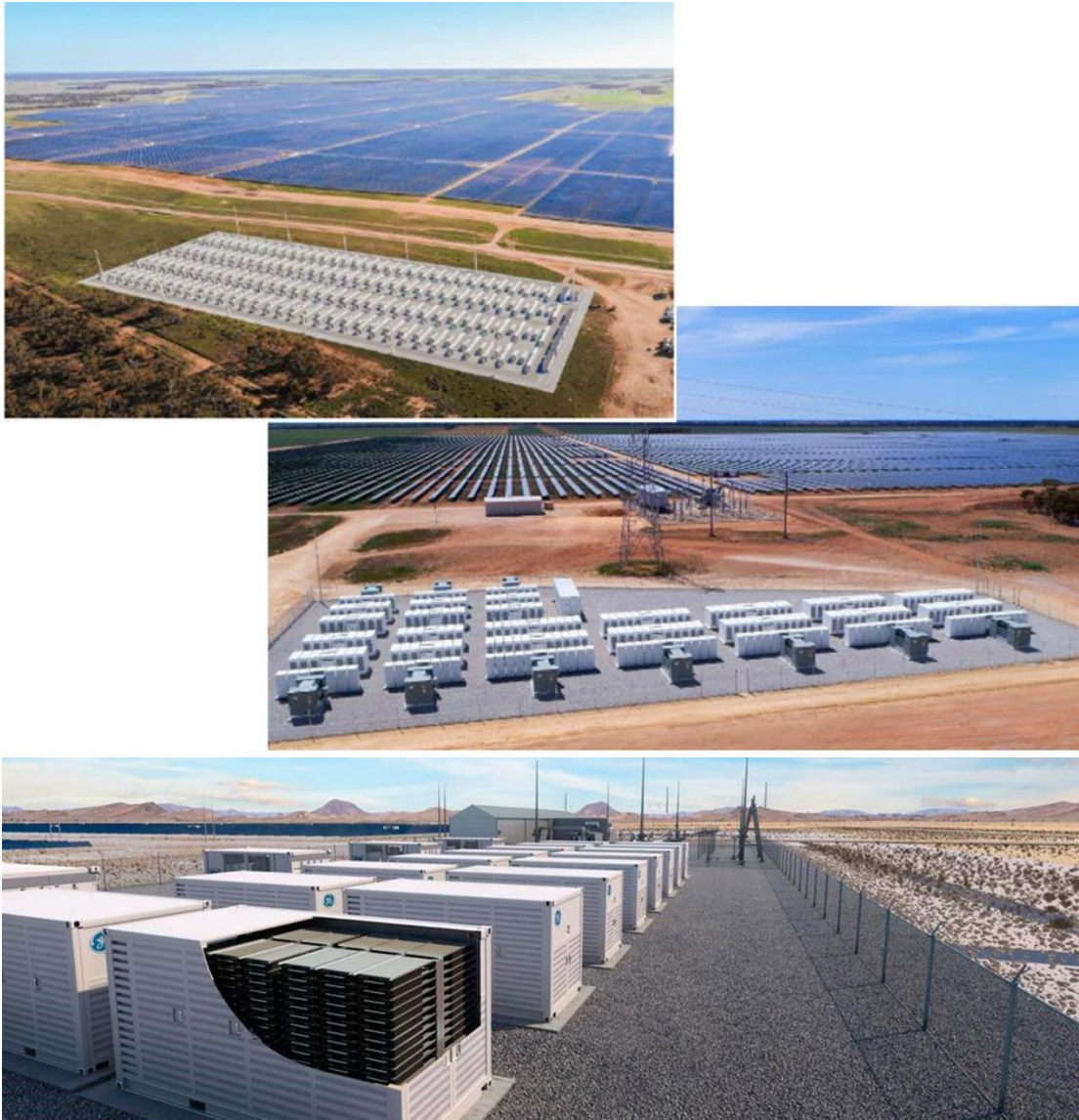
Figure 4-3 – Images of Typical BESS Systems
