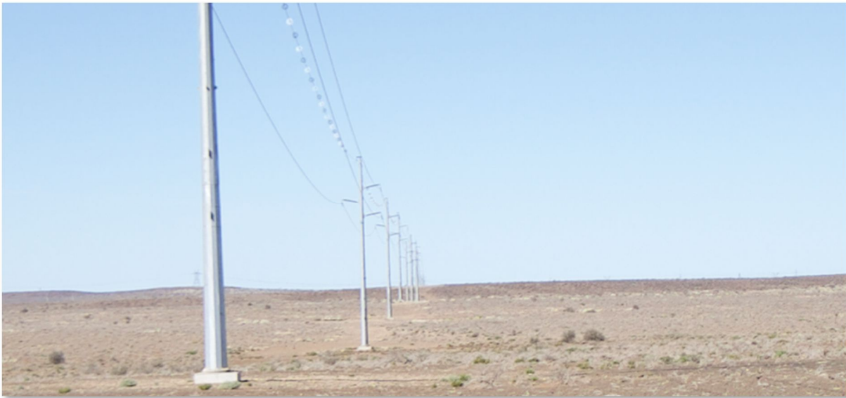
Figure 4-4: The existing 132kV OHL connecting the existing Khobab Substation to the Helios MTS. Lat -30.437863°; Long 19.557748°; Direction SE.
