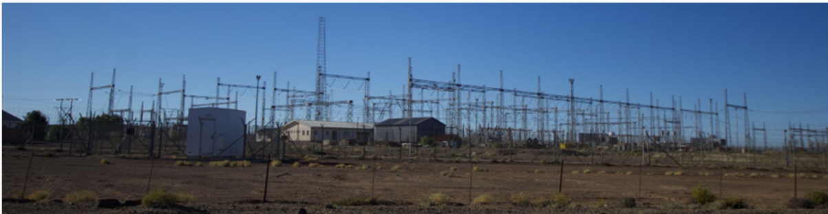
Figure 4-1: Helios MTS where the proposed Kokerboom 4 WEF will connect into the national Eskom grid via the existing transmission line from the Khobab substation to the Helios MTS. Lat -30.497891°; Long 19.557375°; Direction E.
