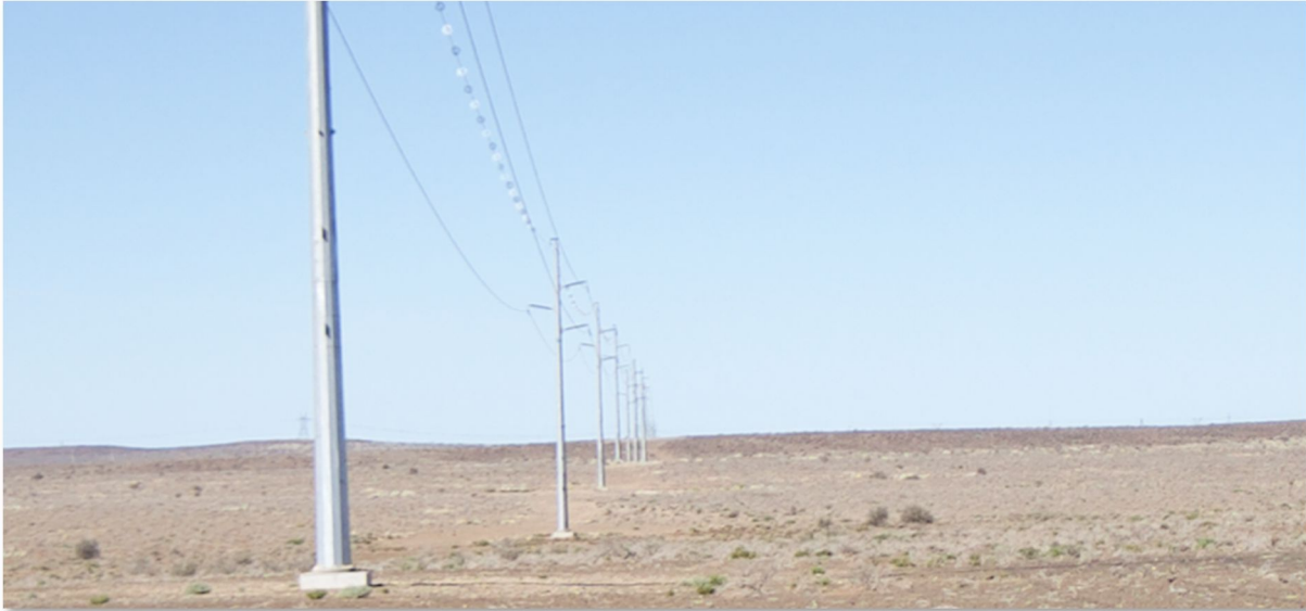
Figure 4-5: The existing 132kV OHL connecting the Khobab Substation to the Helios MTS. Note the spiral line markers (bird flight diverters) to reduce power line collision mortalities of large birds. Lat -30.437863°; Long 19.557748°; Direction SE.
