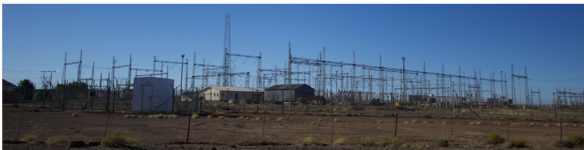
Figure 4-1: Helios MTS where the proposed Kokerboom 4 WEF will connect into the national Eskom grid via the existing transmission line from the Khobab substation to the Helios MTS. Lat -30.497891°; Long 19.557375°; Direction E.
