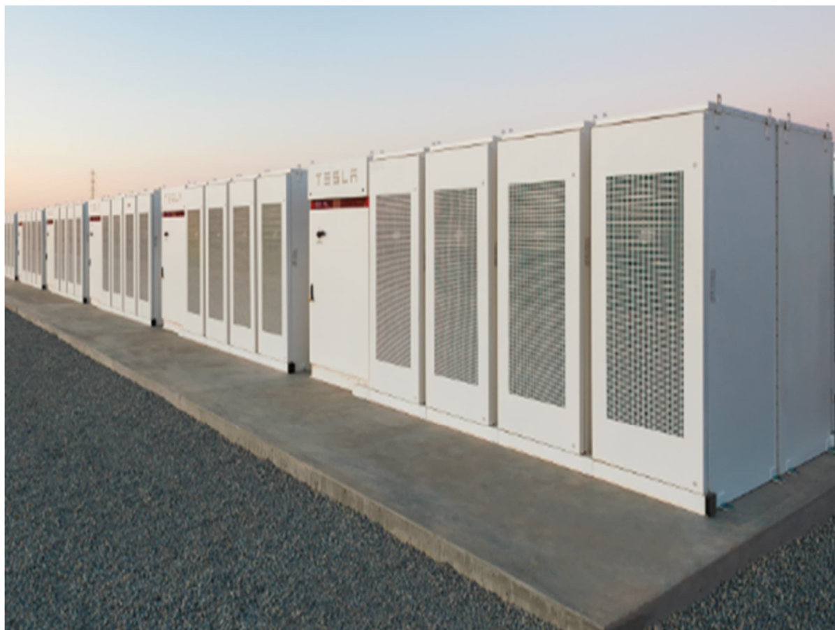
Figure 3-9 Standard BESS Design- Lithium-Ion Solid State Battery
