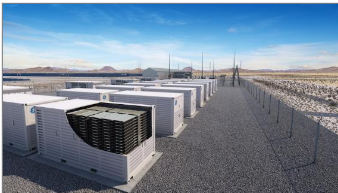
Figure 1: Typical configuration of Lithium-Ion BESS installed inside containers and blocks (Renewable Energy World, 2020)
