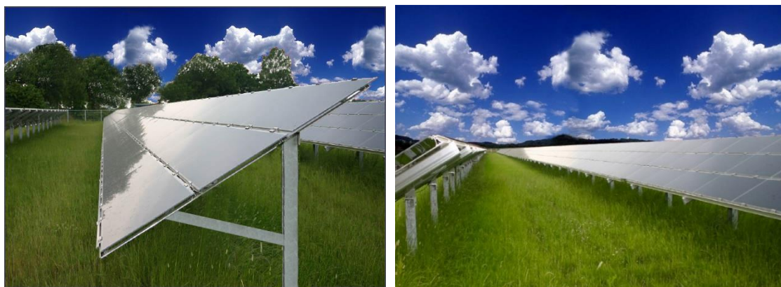
Figure 1-6. Lateral views of PV arrays mounted on fixed mounting systems.
