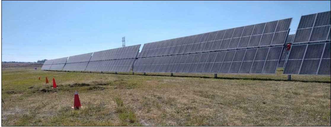
Figure 1-9. Frontal views of PV arrays mounted on fixed mounting systems.
