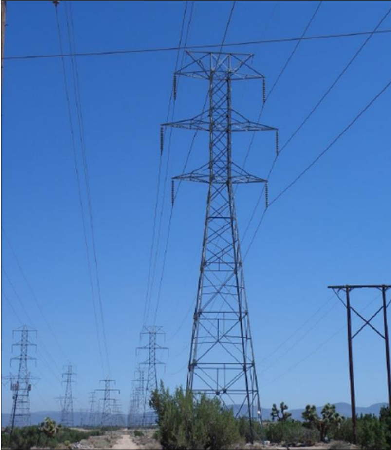
Figure 5-9: 132kV/275kV powerline double circuit suspension towers
