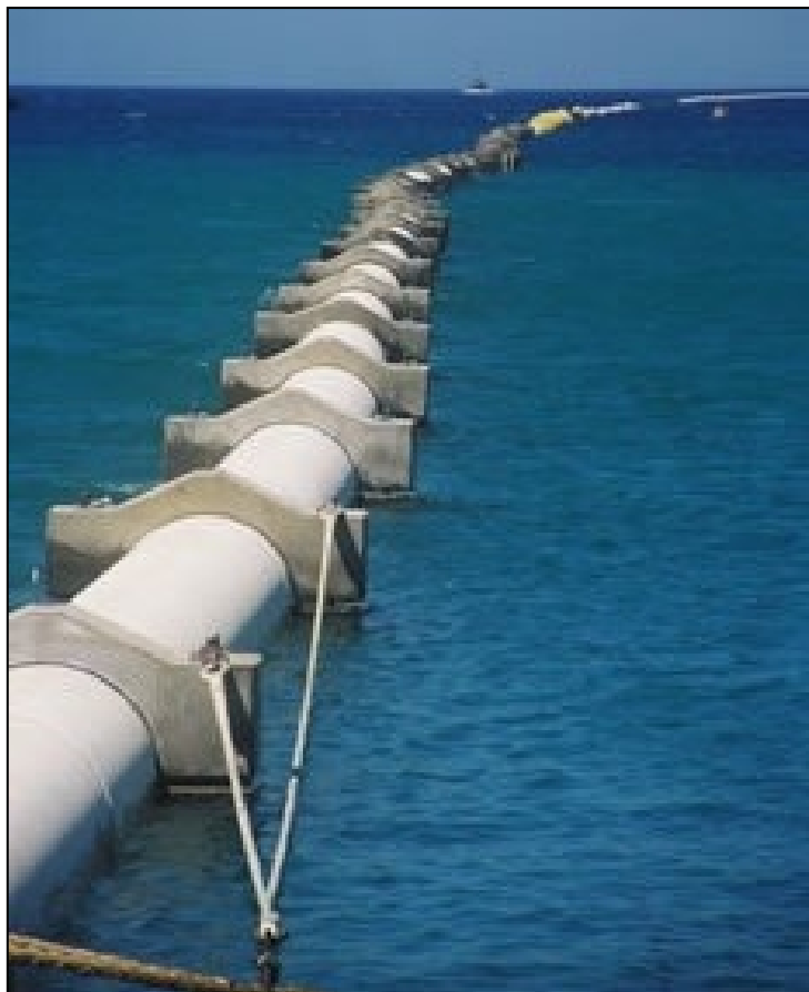
Plate 2.8: Example of effluent discharge pipeline with concrete collars prior to sinking to the seabed.
