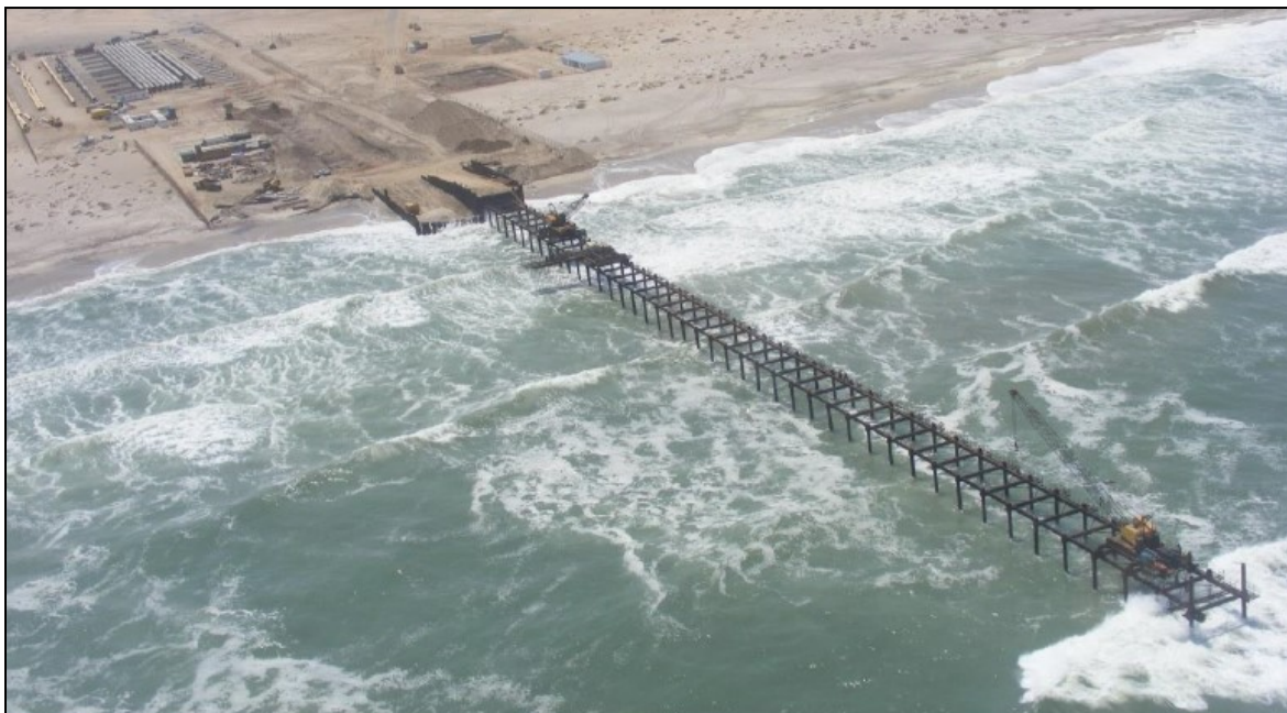
Figure 2.10: Sheet pile jetty structure to provide access for cranes to excavate pipe burial trench (WSP, 2020).
