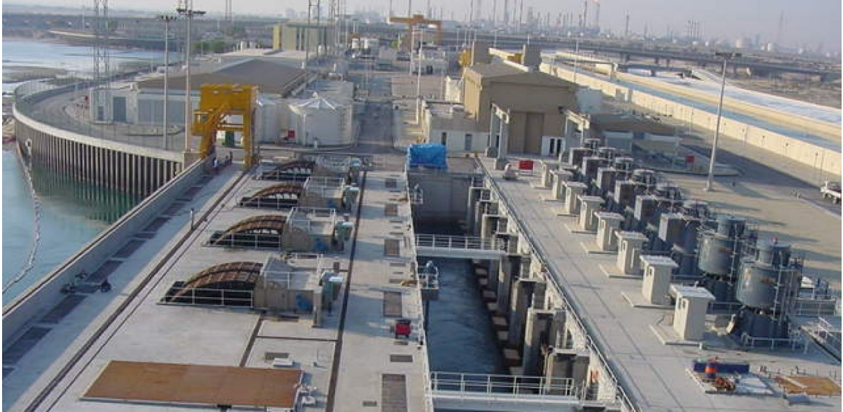
Plate 2.2: Examples of once-through cooling seawater intake infrastructure with vertical pumps on the right (Fluor, Saudi Arabia).
