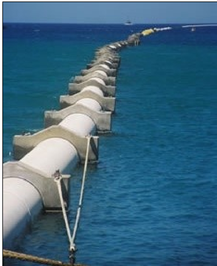
Plate 2.8: Example of effluent discharge pipeline with concrete collars prior to sinking to the seabed.
