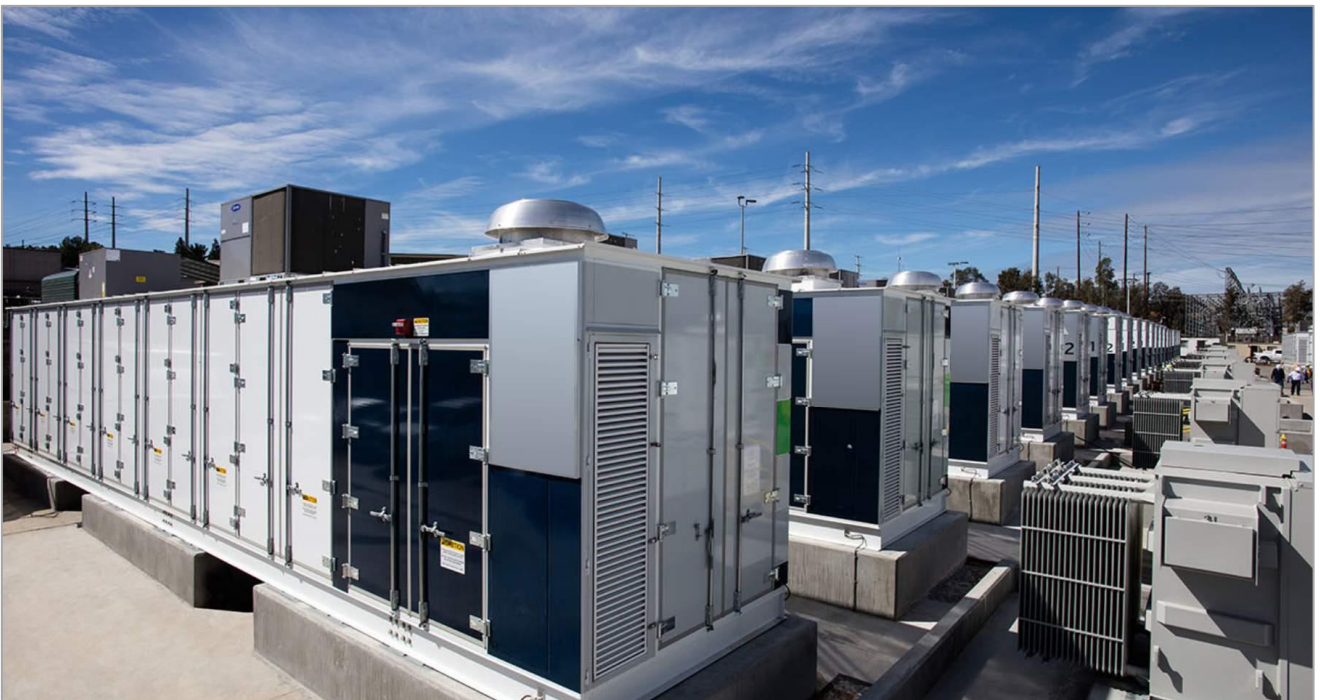
Figure 19: Example of BESS installation ( https://biiworld.com/ )
