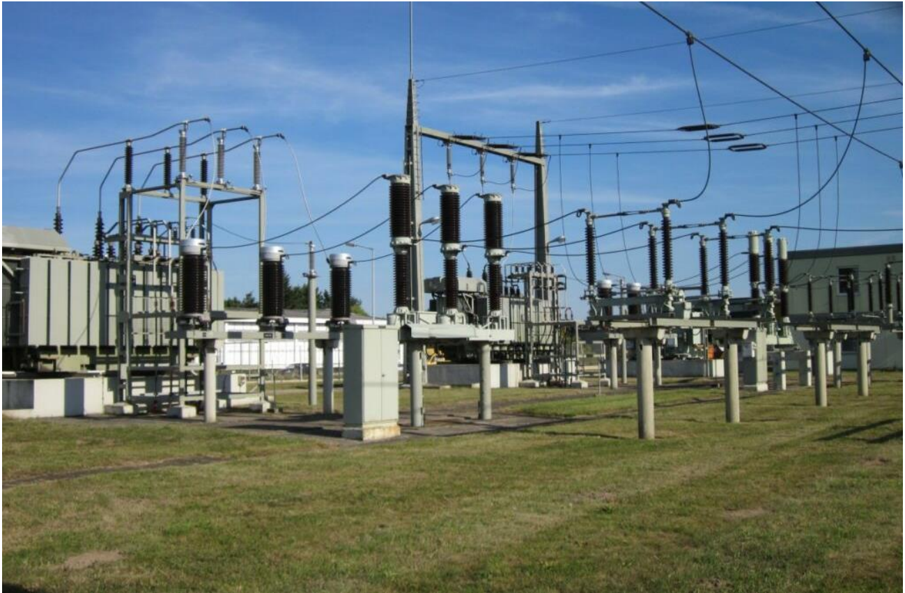
Figure 15: Example of High Voltage Substation
