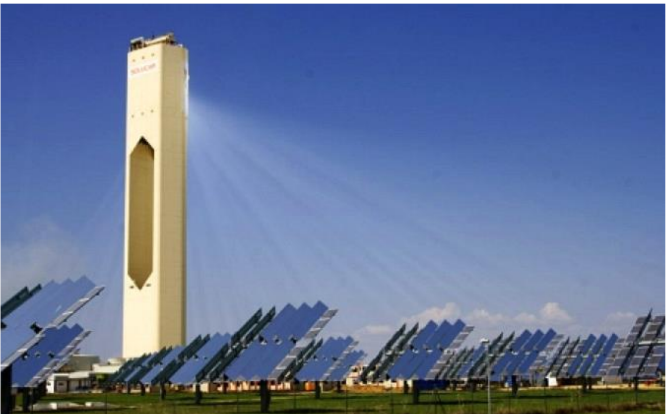
Figure 8: Power Tower Technology (Planta Solar 10, Spain)
