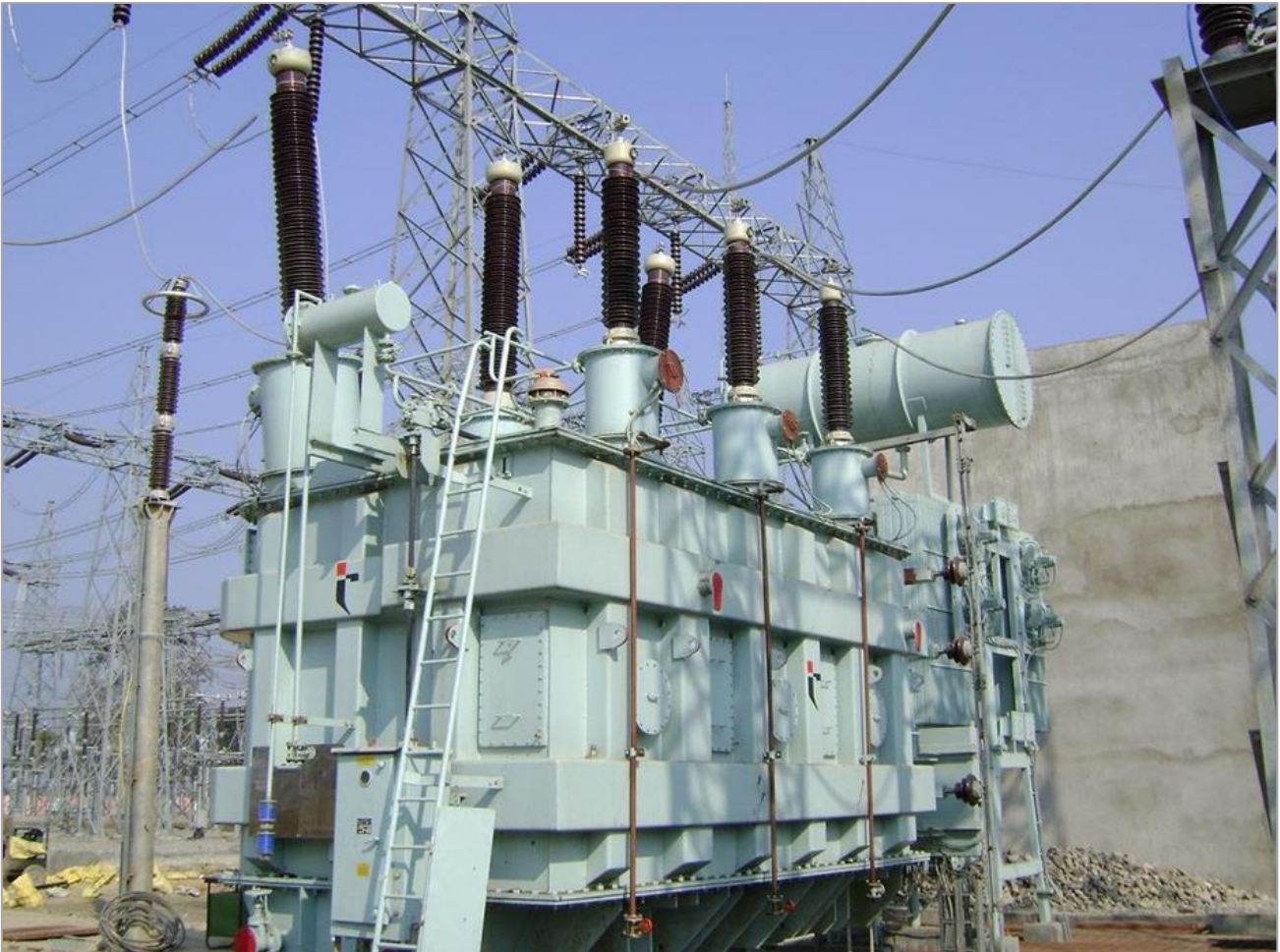
Figure 14: Example of Medium Voltage Transformer
