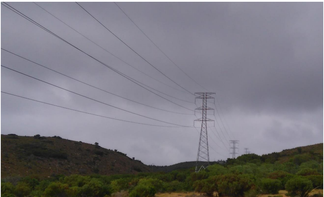
Figure 20: Example of a 132kV transmission line
