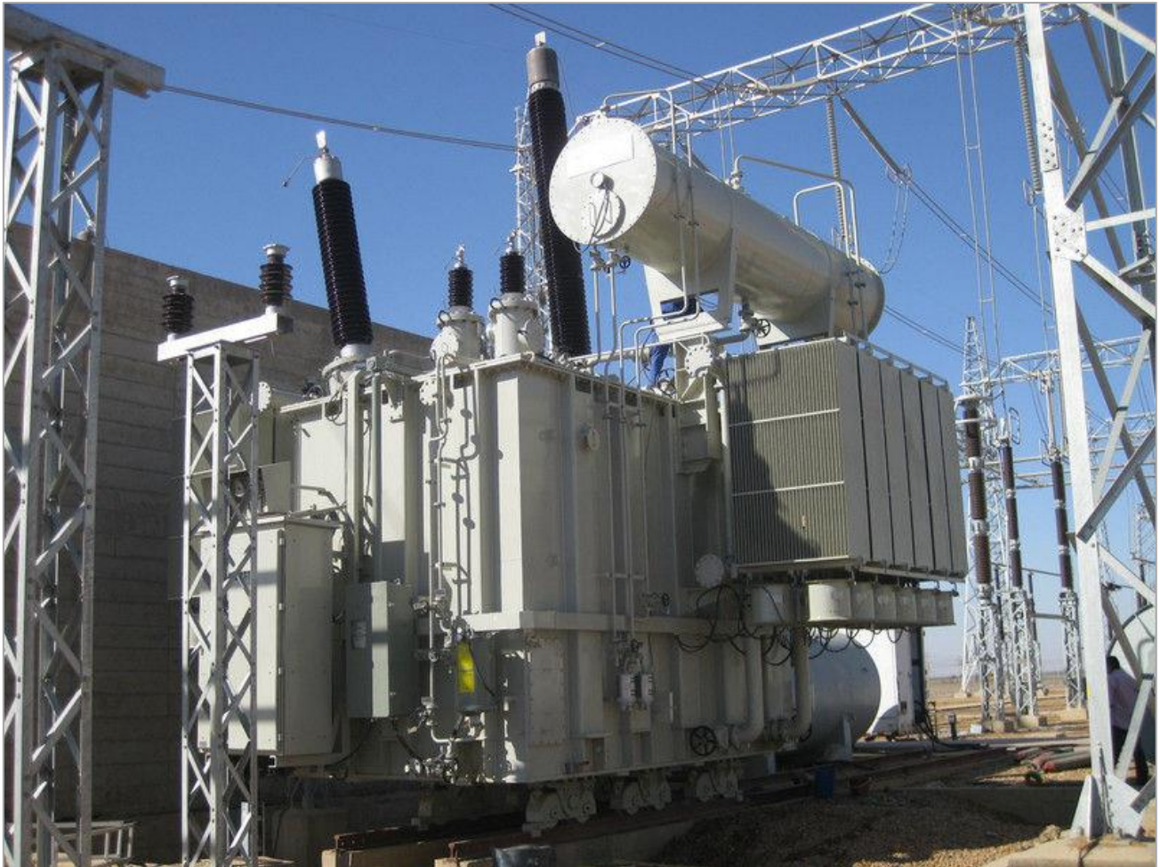
Figure 16: Example of High Voltage Transformers (source: https://www.electricityforum.com/ )
