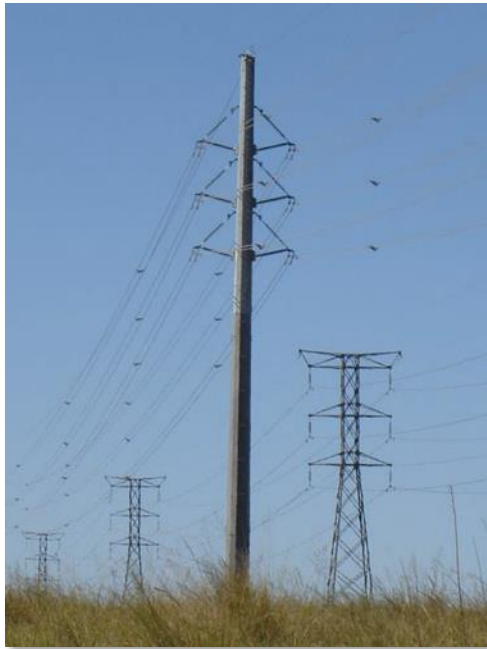
Figure 3: Example of a Self-supporting Monopole (foreground) and Lattice Structure (background)
