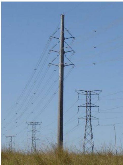
Figure 4-5: Example of a Self-supporting Monopole (foreground) and Lattice Structure (background)
