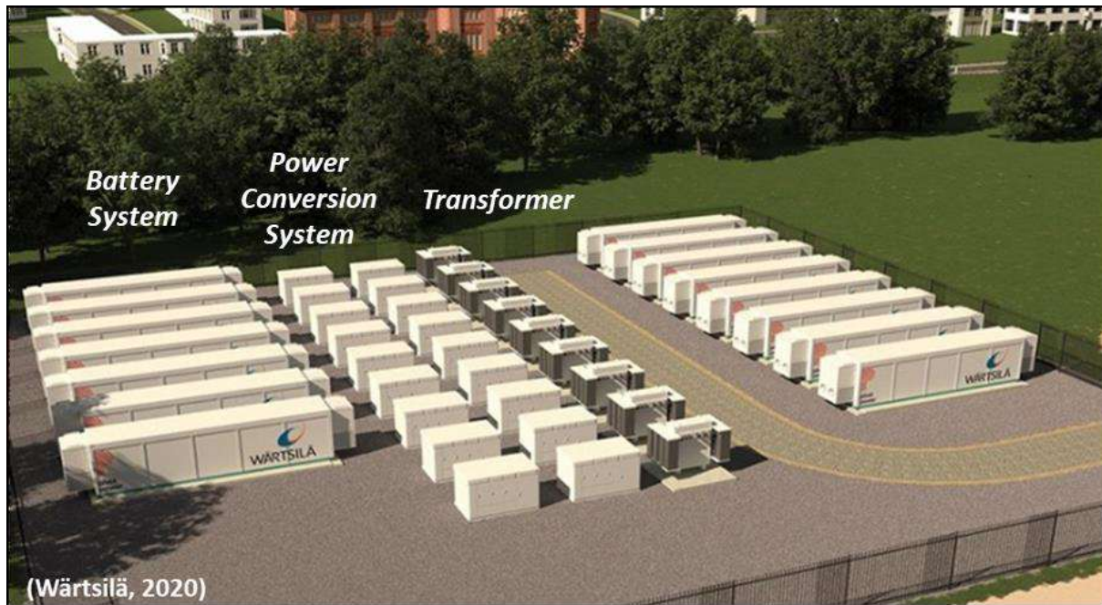
Figure 6: Example of a typical Battery Energy Storage System - Pivot Power's proposed lithium-ion battery in Kemsley, Kent.
