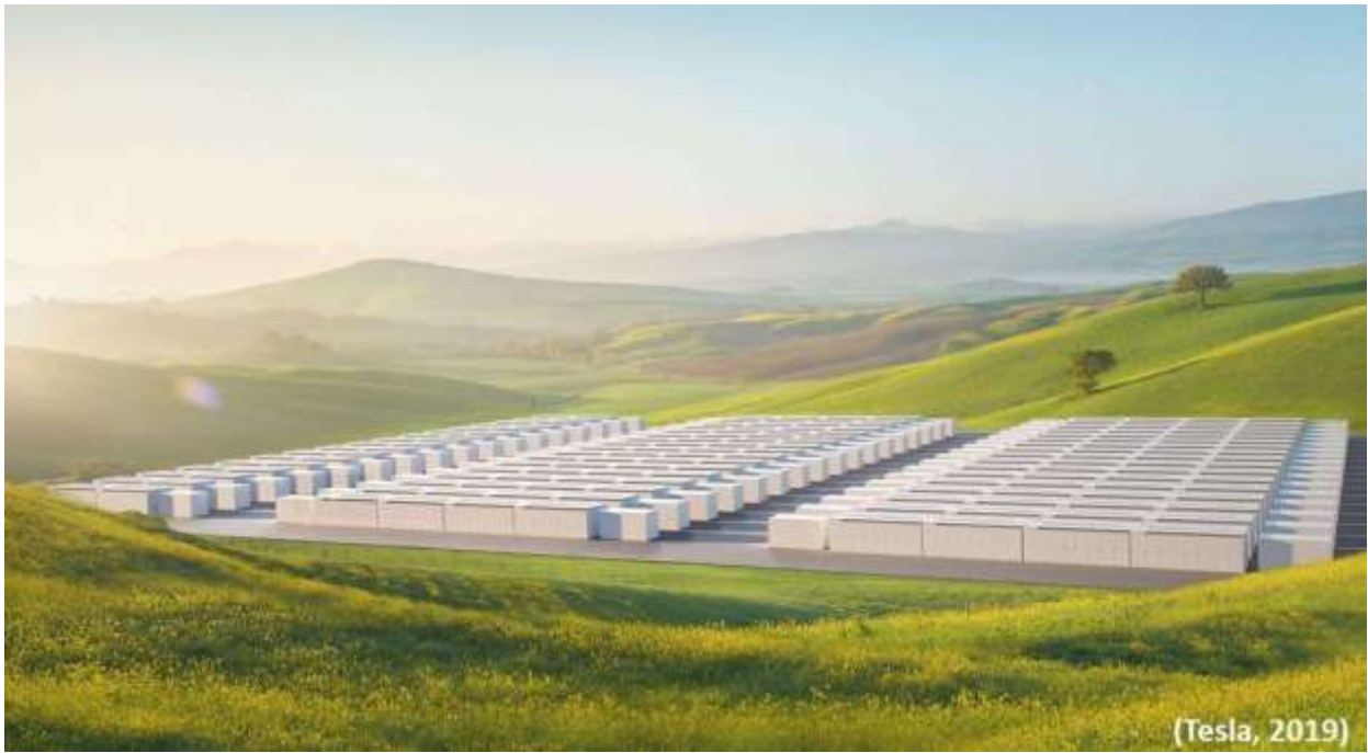
Figure 2: Tesla's Megapack Li-ion Battery (Modular System).
