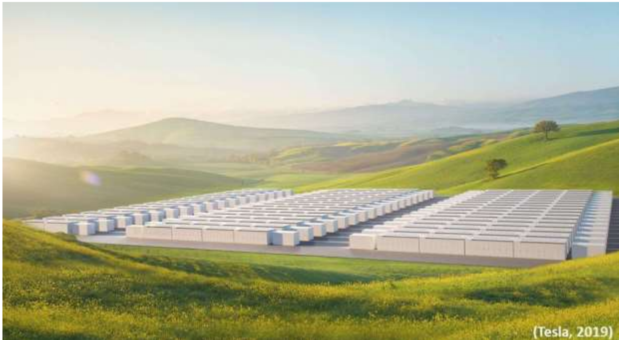
Figure 2: Tesla's Megapack Li-ion Battery (Modular System).
