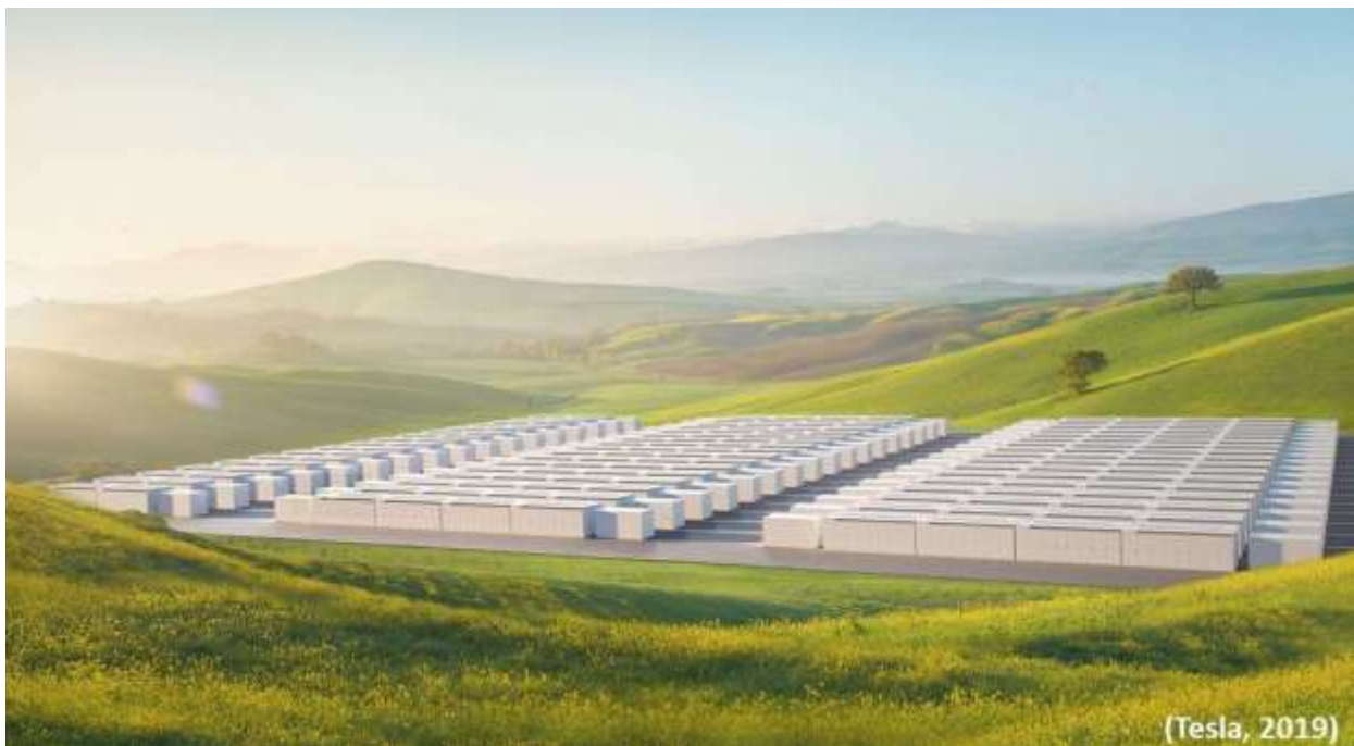
Figure 1: Tesla's Megapack Li-ion Battery (Modular System).
