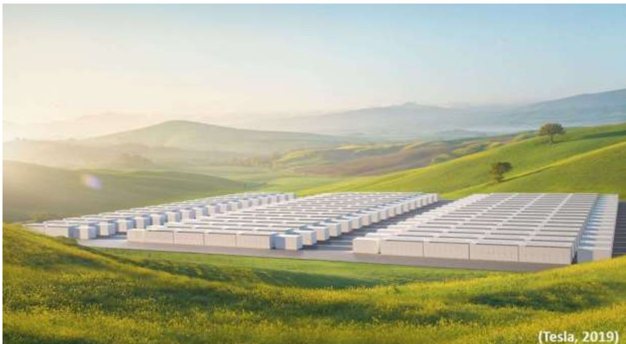
Figure 1: Tesla's Megapack Li-ion Battery (Modular System).
