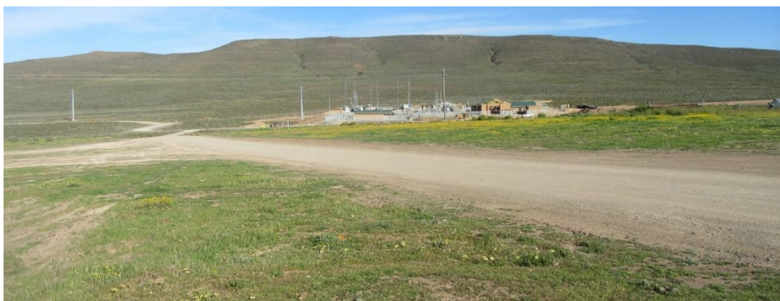
Figure 6-58: Roggeveld WEF substation on Bon Espirange viewed from near the farmstead located to the north-west
