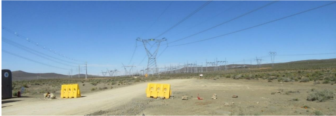
Figure 6-59: Eskom's Komsberg substation, viewed from the entrance along the Komsberg Road
