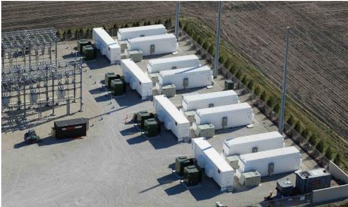
Plate 7-7: A stock image of a similar development with an on-site substation and BESS.
