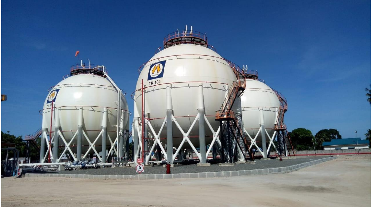
Figure 11: Sphere storage tanks
