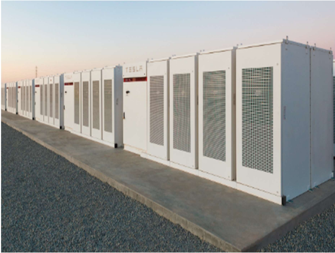
Figure 3-9 Standard BESS Design- Lithium-Ion Solid State Battery
