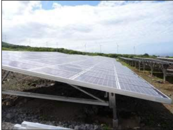
Figure 10: Fixed Solar PV Panels
