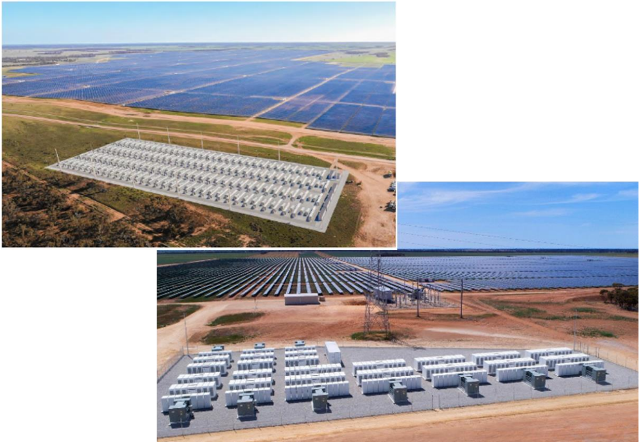
Figure 7-51 – Images of Typical BESS Systems Servicing Solar Power Farms
