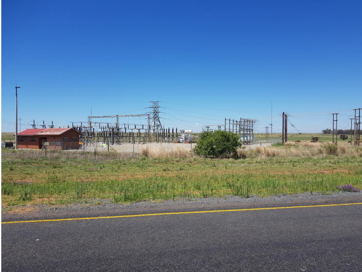
Figure 26: Existing Eskom substation as viewed from the R723 looking south.
