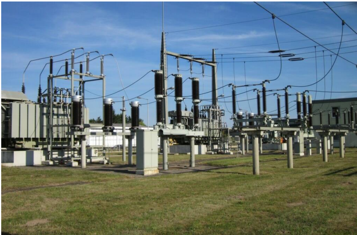
Figure 14: Example of High Voltage Substation (source: https://www.protoenergy.com/ )
