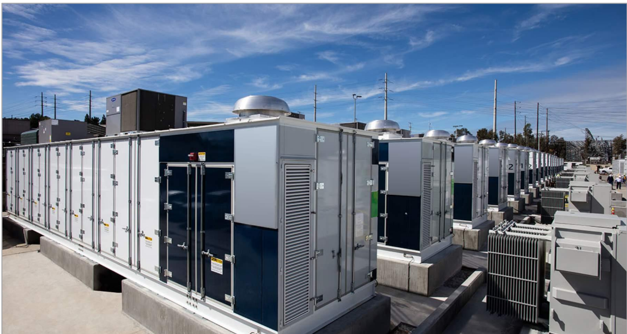
Figure 18: Example of BESS installation ( https://biiworld.com/ )
