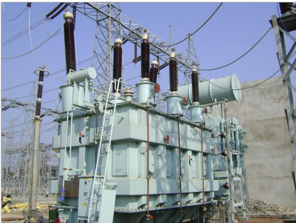
Figure 13: Example of Medium Voltage Transformer (source: https://www.ulaginoli.com/ )
