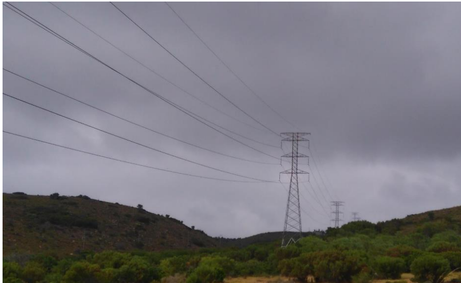
Figure 19: Example of a 132 kV transmission line
