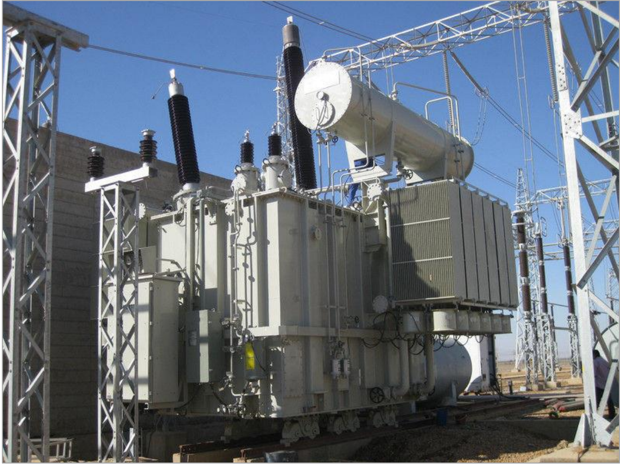
Figure 15: Example of High Voltage Transformers
