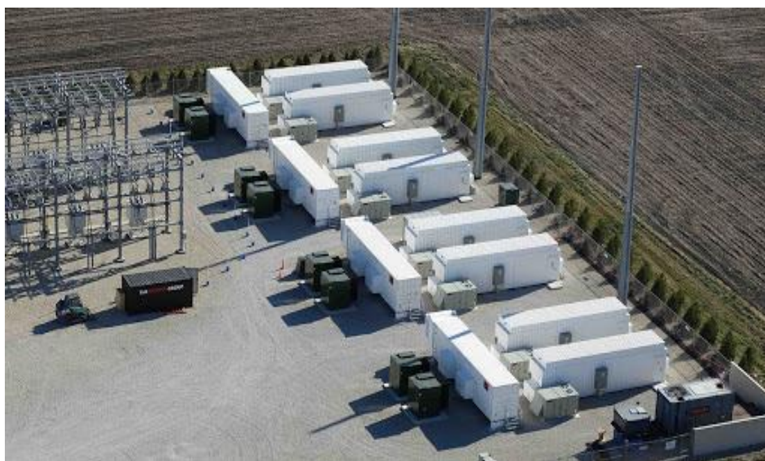
Plate 3-4: A stock image of a similar development with an on-site substation and BESS. Source [ https://reneweconomy.com.au/why-grid-based-battery-storage-is-already-a-no-brainer-in-australia-85967/ ]
