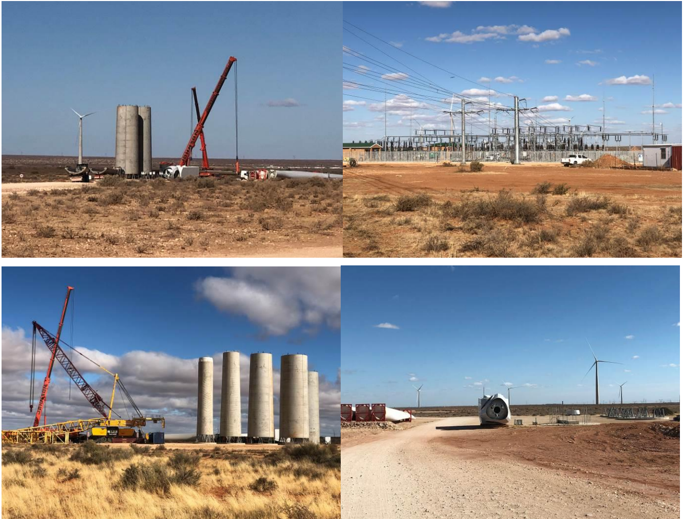
Figure 2-3: Photographs depicting the construction phase of a wind farm similar to De Rust South WEF.
