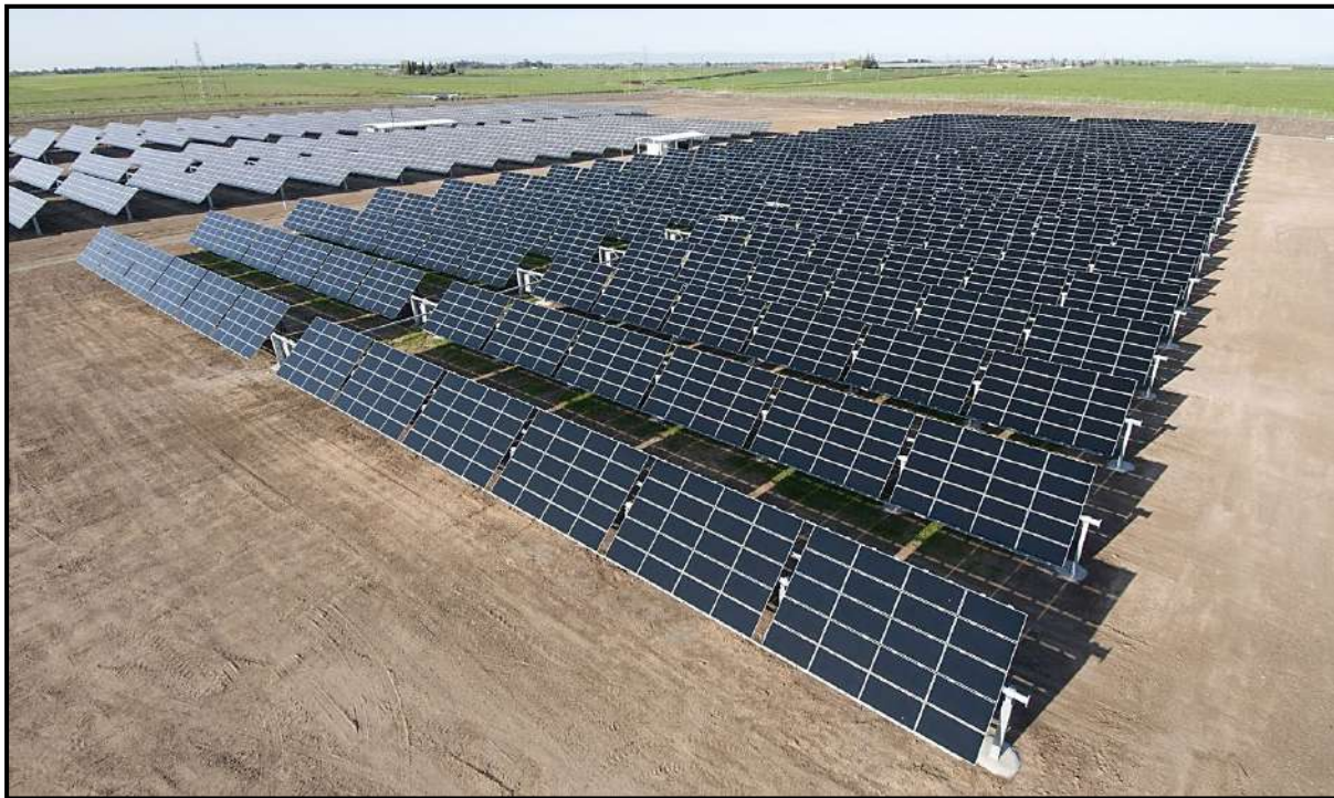
Figure 11 An Array of PV Panels once Mounted
