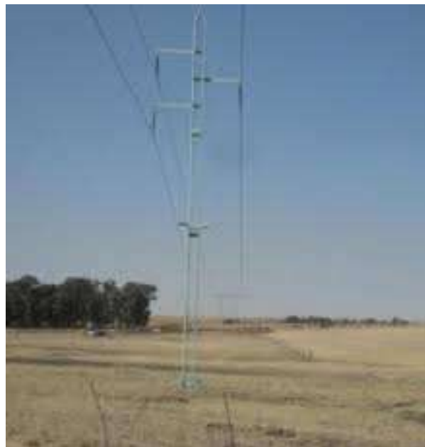
Figure 21: Example of a 132 kV transmission line (steel monopole structure) (SSI, 2012)
