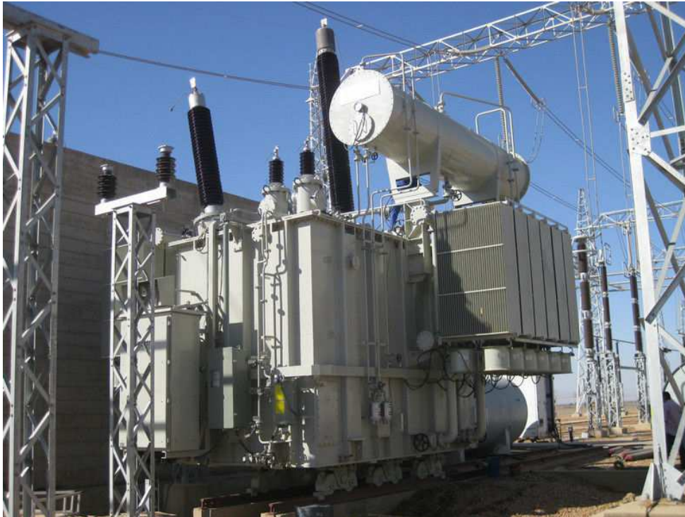
Figure 15: Example of High Voltage Transformers
