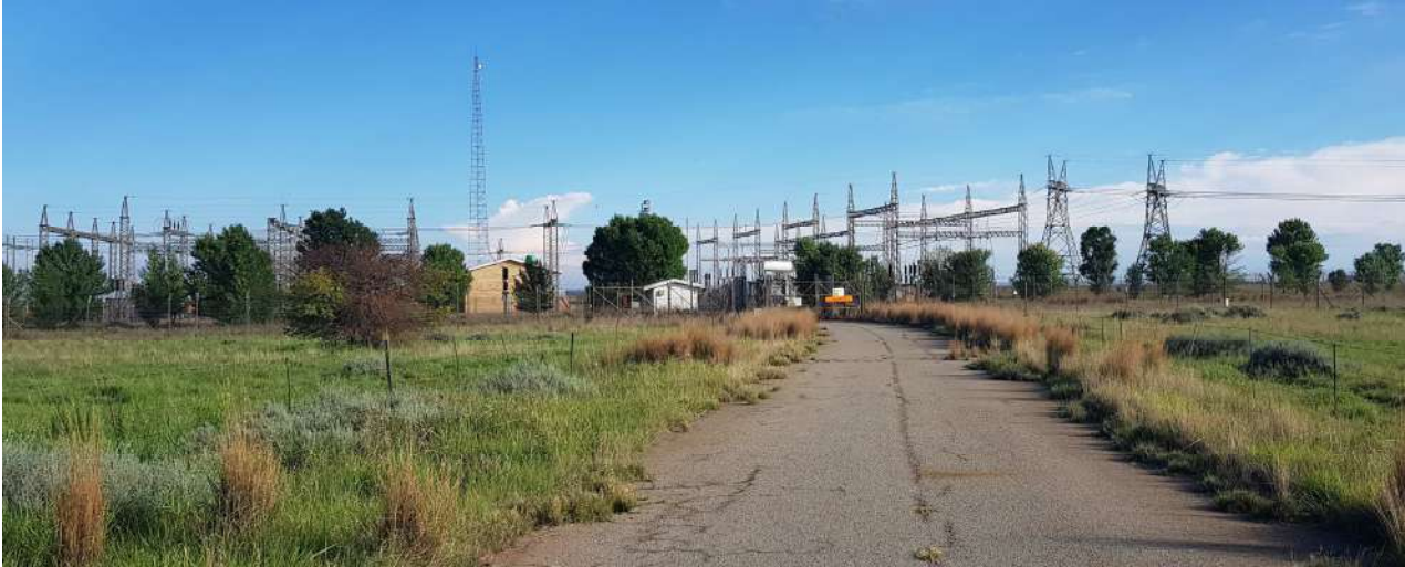
Figure 18: Northern view of the Jersey Distribution Substation
