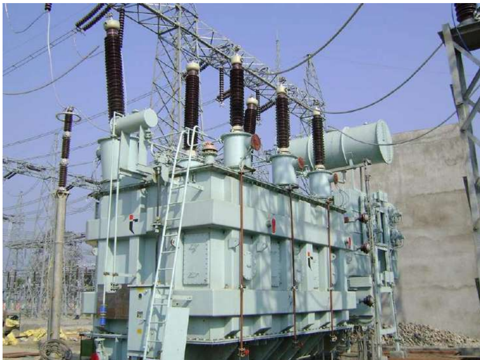
Figure 13: Example of Medium Voltage Transformer (source: https://www.ulaginoli.com/ )
