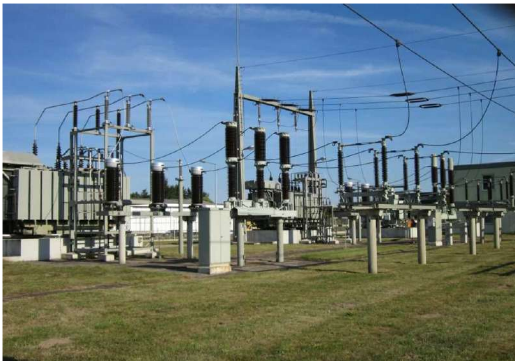
Figure 14: Example of High Voltage Substation
