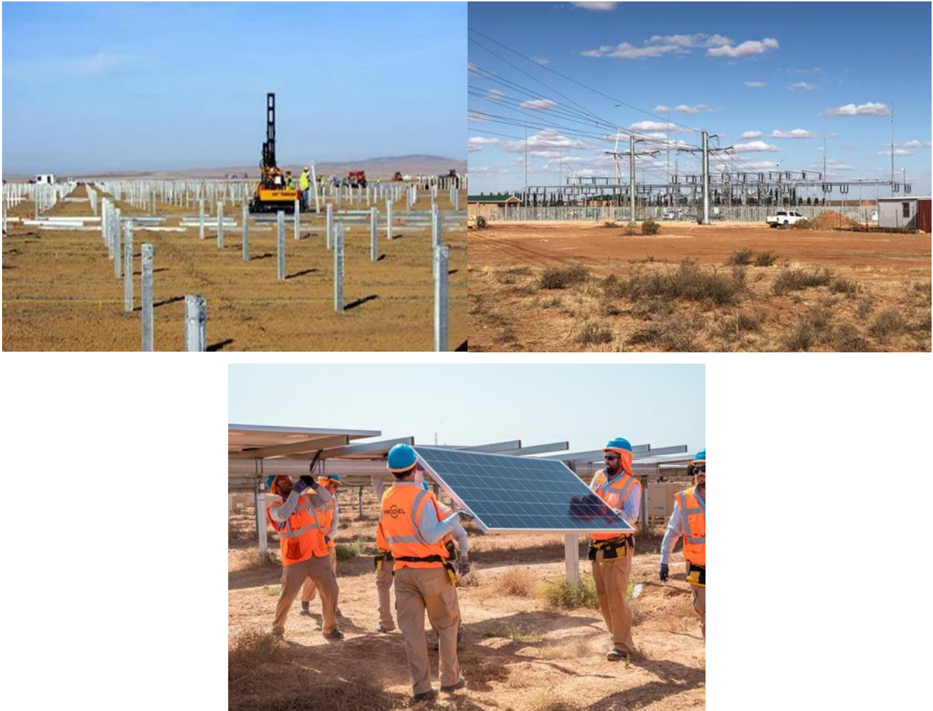
Figure 2-4: Photographs depicting the construction phase of a solar farm similar to De Rust PV1 SEF. Source: www.power-technology.com , renewablesnow.com .
