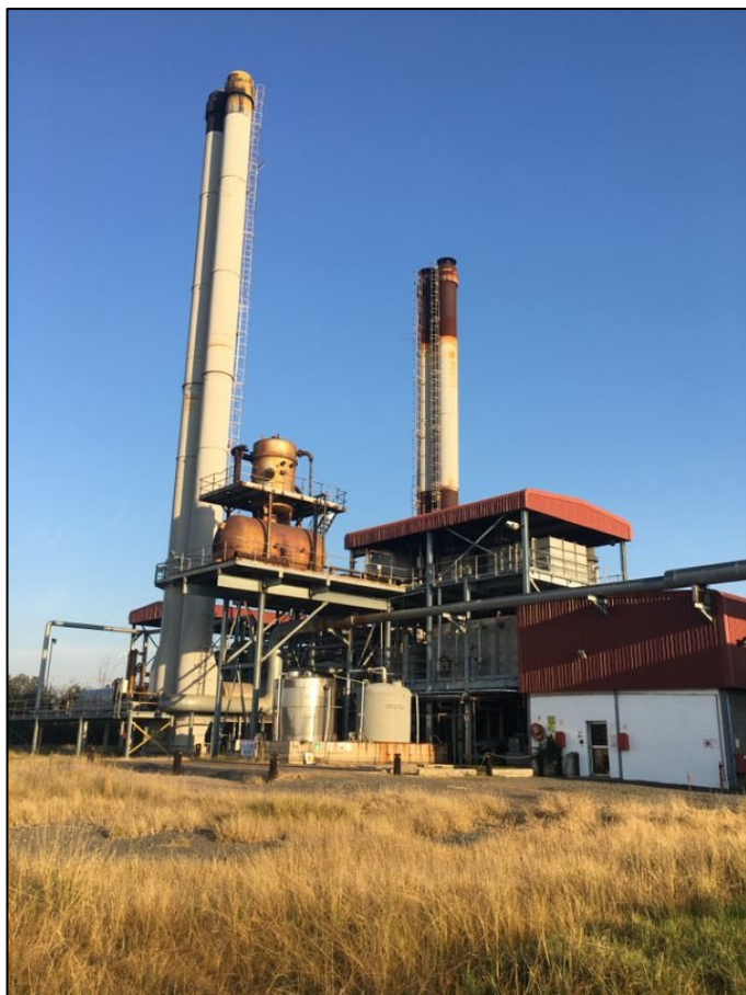
Figure 6-1 (a): View of cogeneration plant
