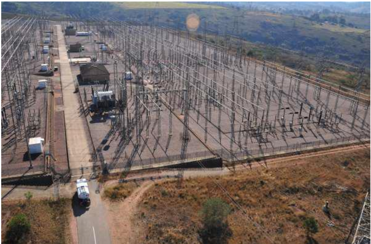
Figure 4: Typical substation site
